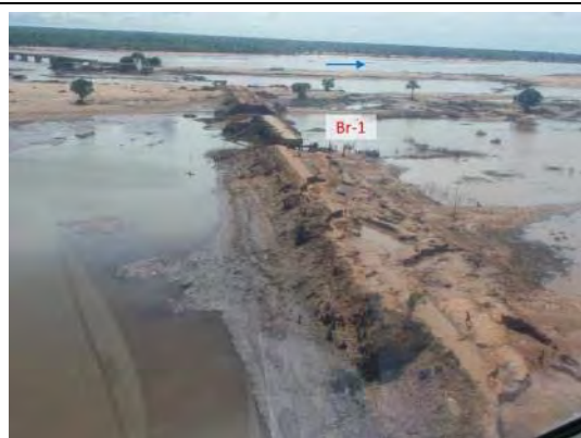
Approach road to Br-1: Crown of embankment was eroded due to overflow
