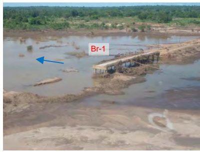
Br-1: Main body is remained but approach roads of the both side were washed away
