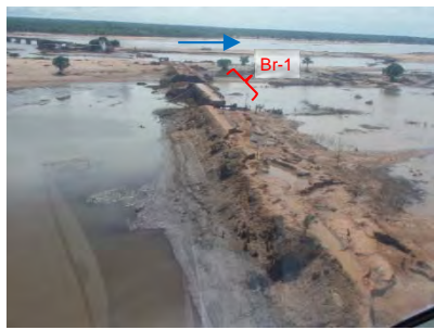
Approach road to Br-1: Crown of embankment was eroded due to overflow
