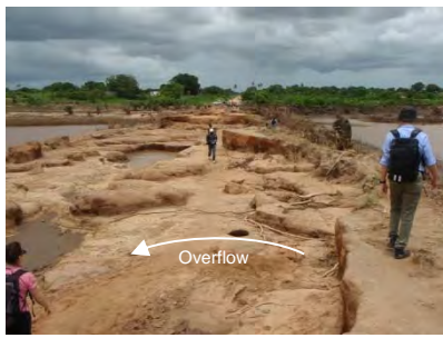
Approach road to Br-1: Crown of embankment was eroded due to overflow
