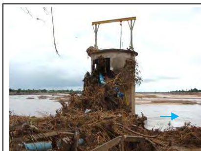
Intake facility for water supply on right bank of Lugela River was damaged
