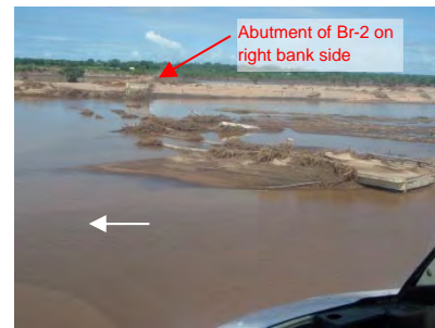
Br-2: Dropped bridge beam
