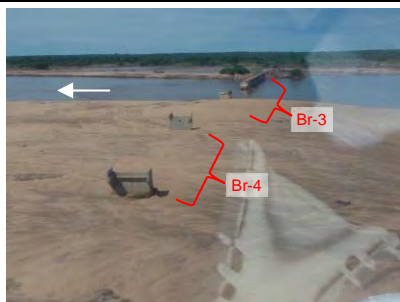
Br-4 (Licungo III): Portions except abutments were washed away and embankment between Br-3 and Br-4 was also washed away
