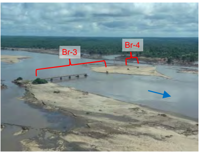
Br-3: 6 spans of right bank side are remained but beams and piers of other 3 (?) spans were washed away
