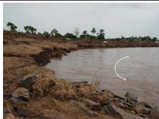
Riverbank erosion at upstream of intake facility. (Lugela River)
