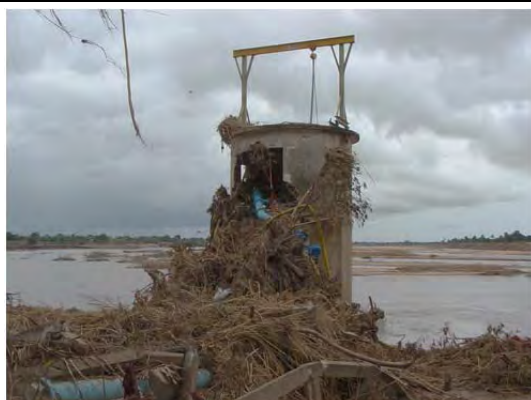
Intake facility for water supply on outer bank of curve reach was damaged. (Lugela River)
