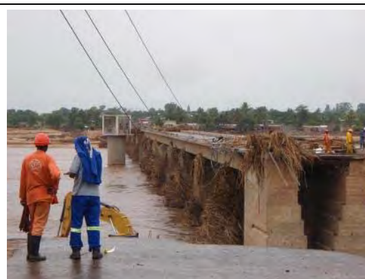
Licungo R. Br: Right bank was eroded but bridge body is remained.
