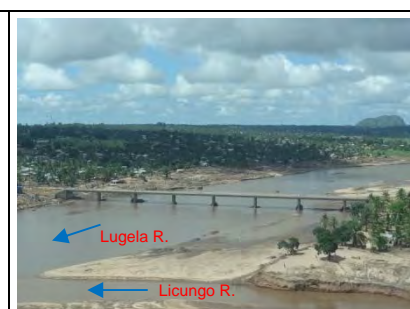
Lugela R. Br: Some railings were washed away due to overflow but traffic is secured after cleaning the debris on the bridge
