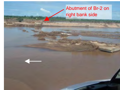
Br-2: Dropped bridge beam
