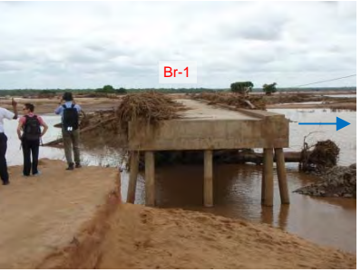
Br-1: Eroded approach road on right bank side
