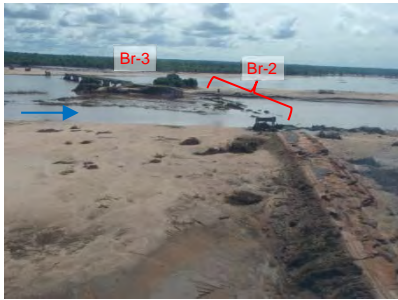
Br-2: Abutments are remained but other portions were washed away
