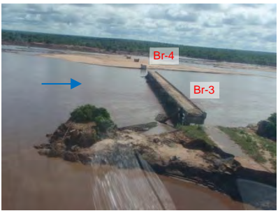
Br-3 (Licungo II): Bank on right bank side was eroded
