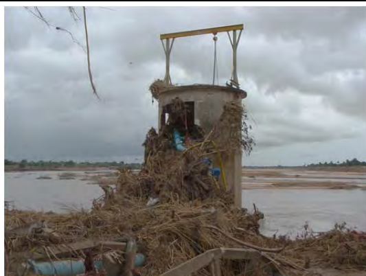
Intake facility for water supply on outer bank of curve reach was damaged. (Lugela River)
