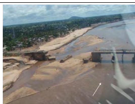
Licungo R. Br: Embankment at left bank side was washed away and a culvert is remained.
