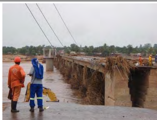
Licungo R. Br: Right bank was eroded but bridge body is remained.
