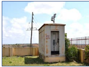
Electric power substation
