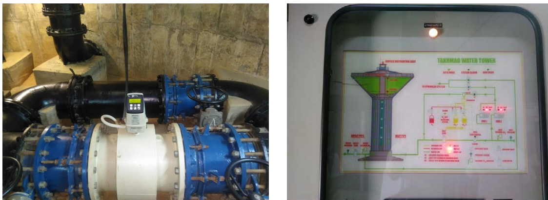
Figure 1-4.9 Monitoring Status of Ta Khmau Existing WTP
