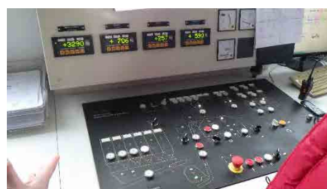
Control panel of concrete plant
