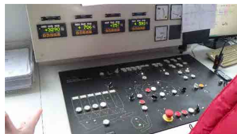
Control panel of concrete plant
