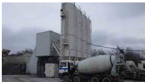
Concrete plant, Cement silo, Agitator truck
