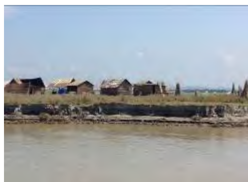
Erosion of the Char Land
