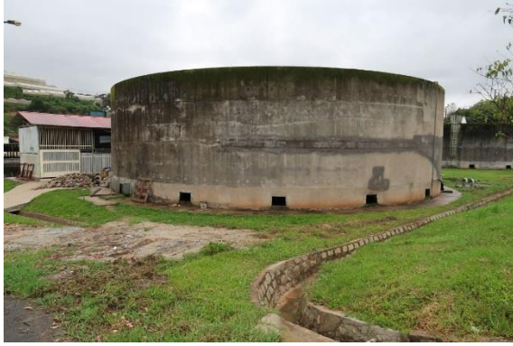
Trickling filter tank
