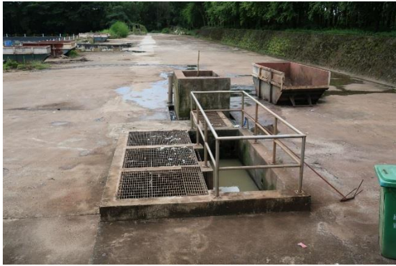
Diversion tank (SB-1)
