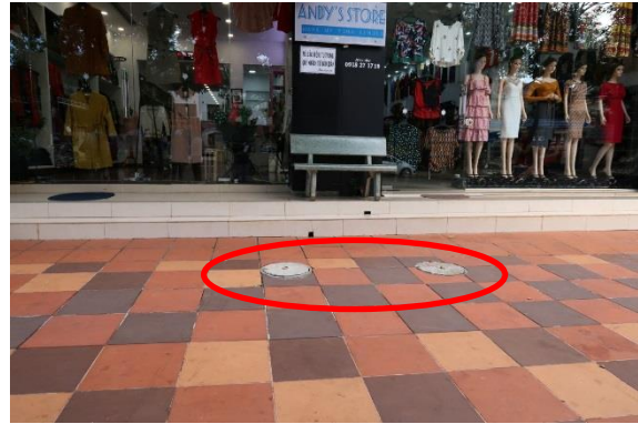
Connection box receiving sewage from the store
