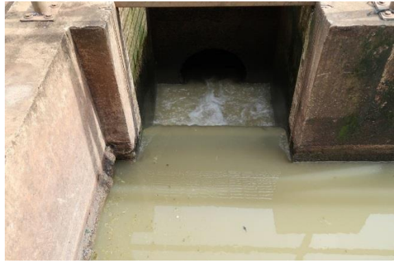
Outlet of diversion tank (SB-1)
