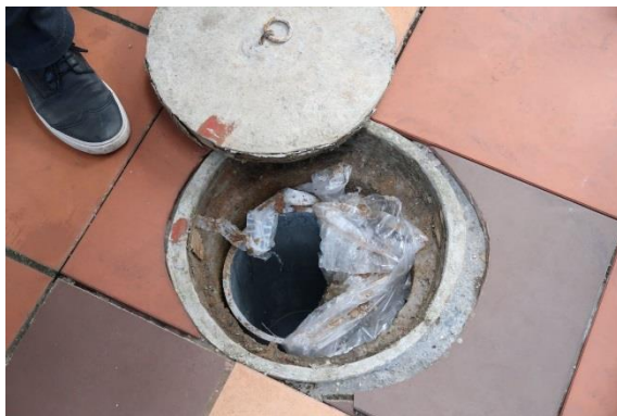
Inside of connection box
