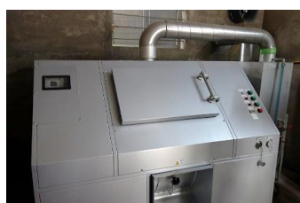
Composting Plant Installed
