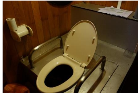
Composting Toilet Installed
