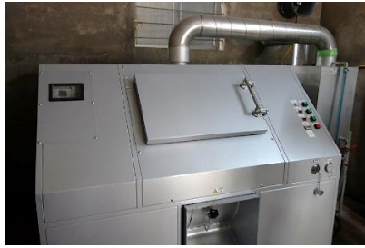
Composting Plant Installed
