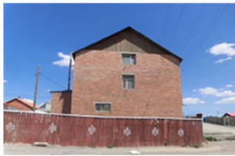
Figure 4 Out-of-plane direction vulnerable building in Mongolia
