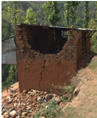
Figure 5. Out-of-plane destruction due to insufficient coupling with the horizontal plane
