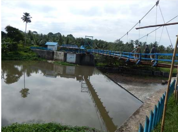
Water Vang Head Work (Tughumulyo Irrigation System)
