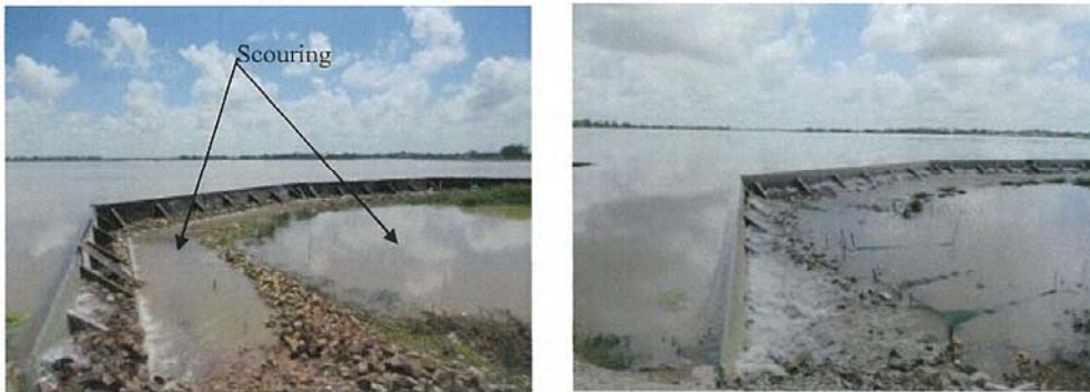
Figure A8-1 Vay Kor Dam During Placing Cobbles (Left) and After Placing Cobbles (Right) against Scouring in the Downstream Side of the Dam
