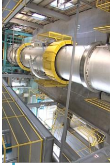
Rotary kiln for mercury waste
