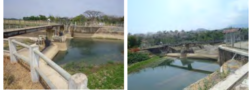
Has Damage at top and must replace ASAP
