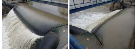
Original Bridgestone Product was 26 year operation but the rubber has damage at crease and must replace
