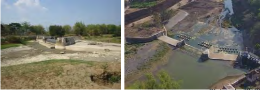
Has blow up at center of RD on 1year ago. Change to fixed weir and make 55m river widening Picture by PUPR
