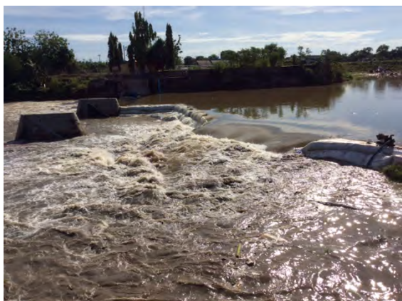
写真-3: 仮締切決壊直前 (2017/11/8)
