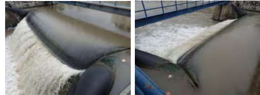
Original Bridgestone Product was 26 year operation but the rubber has damage at crease and must replace
