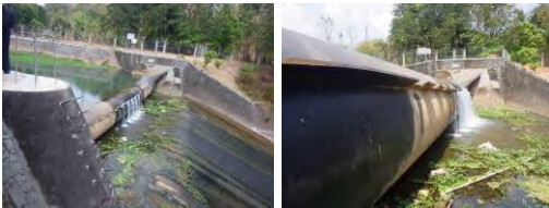
Original Bridgestone has Functional but only a few year to operation (must replace)
