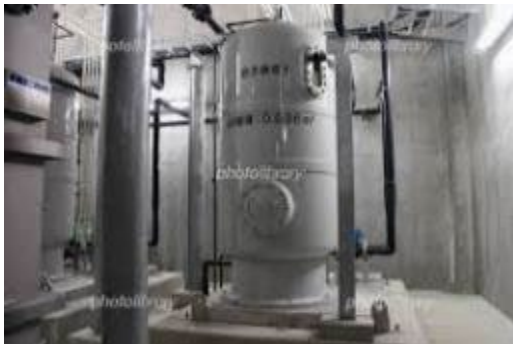
Sand filtration treatment (physicochemical treatment process)
