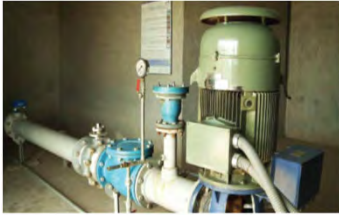
Air and check Valves
