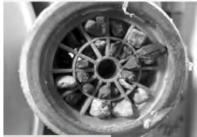
PARTIAL CLOGGING CAUSED BY SUSPENDED PARTICLES
