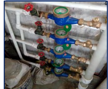
Water Meter at Building
