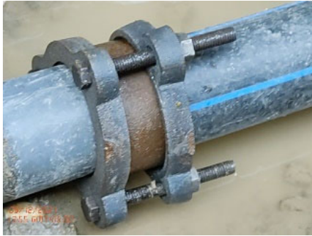
Connection between PVC and HDPE
