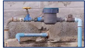
Water Meter at House
