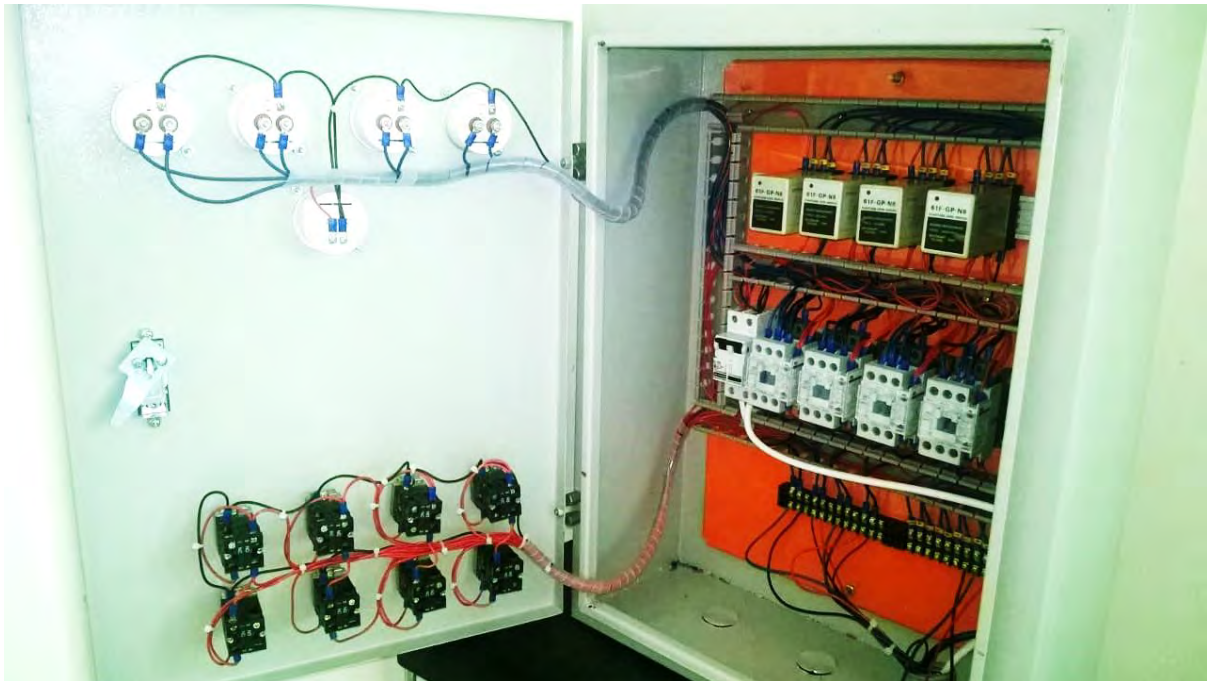
(DOL panel for miniature Pump Station)
