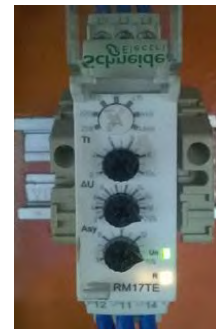
Phase Failure Relay
