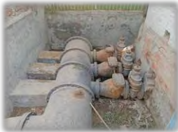
Discharge Valve & Check Valve
