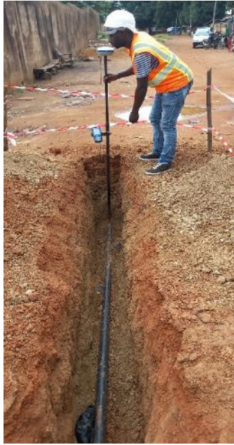
Tuyau PVC 63 mm alimentant la station de purification
