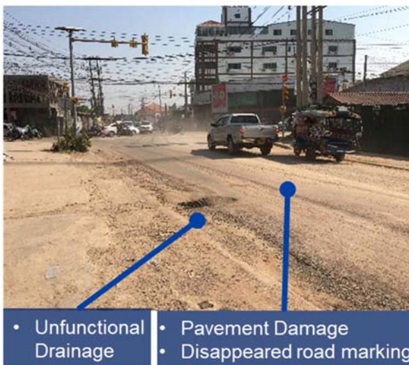
Figure 12.2-14 Road Condition in Vientiane Capital
