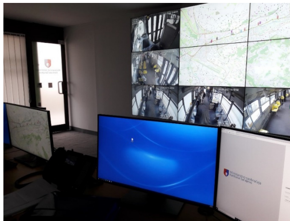
Figure 2.4.2 Traffic Control Center in Sarajevo
