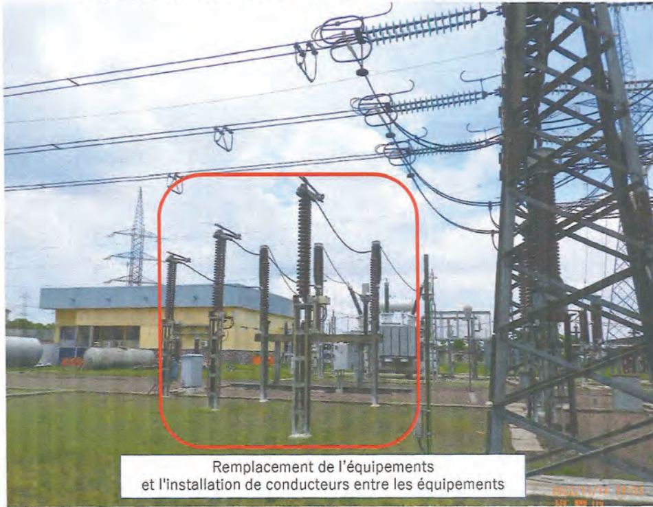
② Appareillages 220kV (travee Tfo-1), LIMINGA
