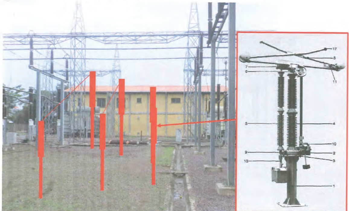
② Appareillages 220kV (travee Tfo-2), FUNA
