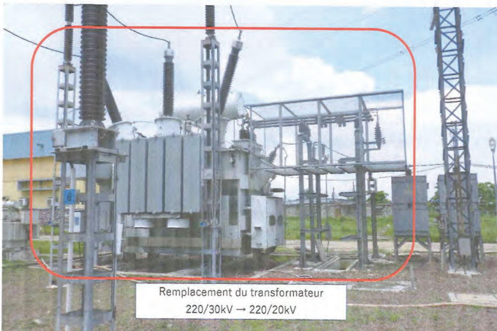
① Tfo-1 (220/20kV, 20/0.4kV), LIMINGA
