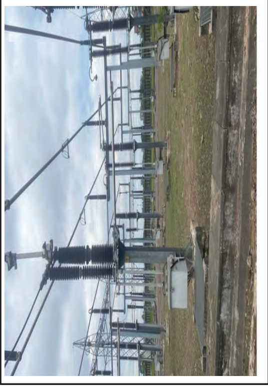
Photo n° 05 : Pantograph disconnector of the Funa substation
