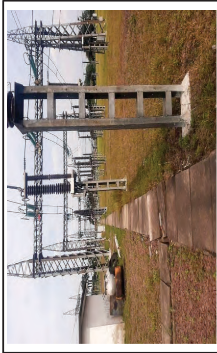
Photo n°04 : One of the technical cable passage gallery
