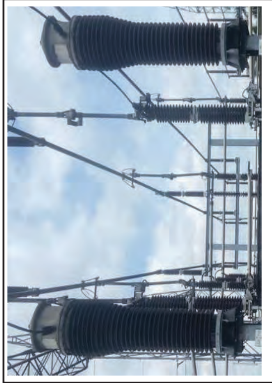
Photo n°06 : Transformation of Intensity (T1) of the Funa substation
