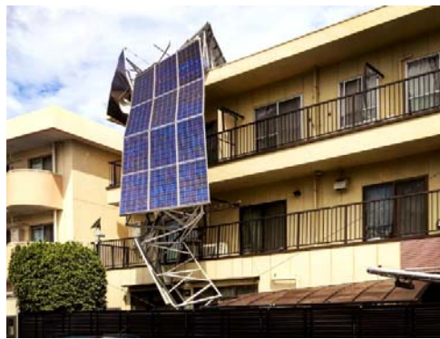
9 Sep 2019 Kanto, Japan @kadowaki_kozo Damage of roof-top structure by high speed wind
