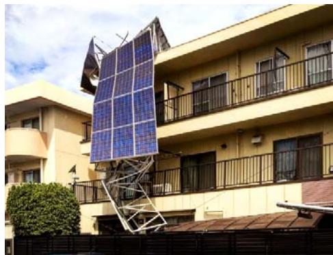
9 Sep 2019 Kanto, Japan @kadowaki_kozo Damage of roof-top structure by high speed wind
