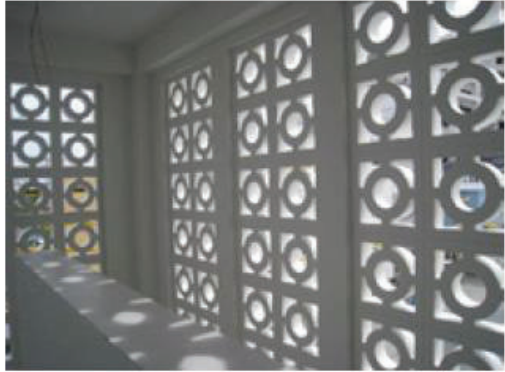
Lighting with utilization of HANA block
