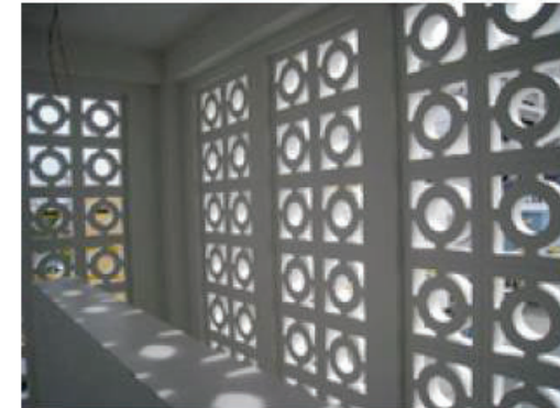
Lighting with utilization of HANA block
