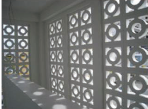
Lighting with utilization of HANA block
