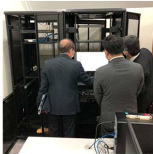
Photo-4 Equipment of Data Centre such as server and data storage
