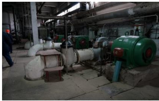
Tashkent City No. 1 combustion air supply fan and gas piping at district heat supply station
