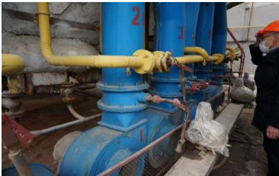
Tashkent City No. 1 combustion air supply fan and gas piping at district heat supply station
