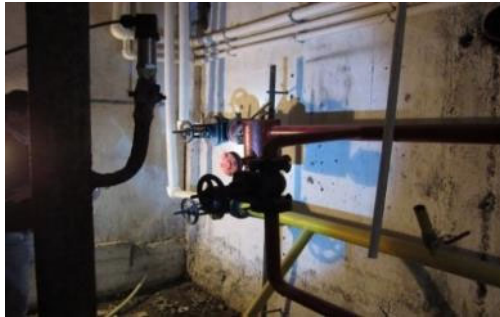
the upper illustration Tashkent City No. 8 Insulation of return water piping at district heat supply plant
