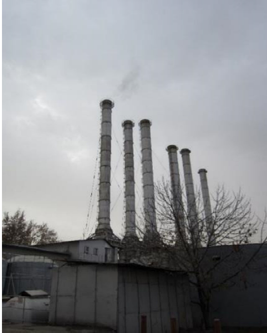
Tashkent City No. 1 combustion air supply fan and gas piping at district heat supply station (Emissions other than water vapor.) The reality of the
