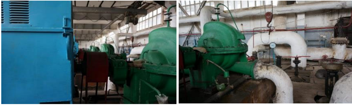
Tashkent City No. 8 hot water supply pumps and electric motors for district heat supply plants
