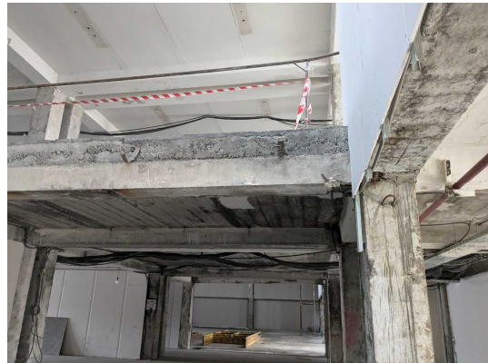
The interior of the renovated building The columns and beams are made of reinforced concrete, and the precast floor slab is placed on top of the beam, with concrete laid on top as a finishing material.
