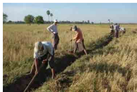
Excavation of water course is carried out by farmers themselves with a support from IWUMD and DOA officers.
