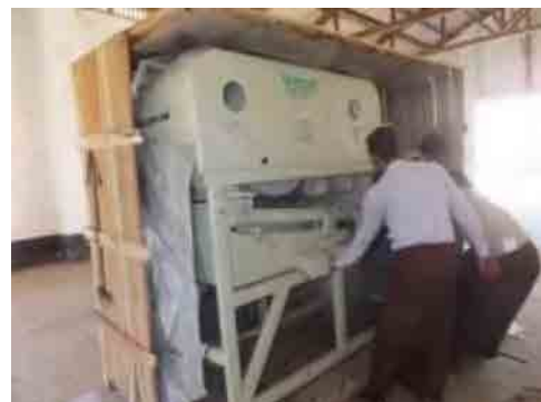
The third seed cleaner from India is being installed in Paundale, Pyay township.
