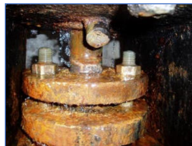
Leak from grand packing
