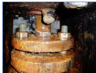
Leak from grand packing
