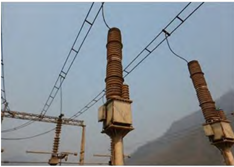
Insulator of circuit breaker and disconnector
