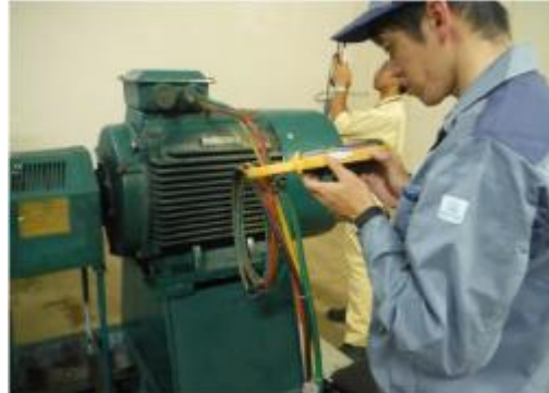
Drain Pump Motor Measurement Scene
