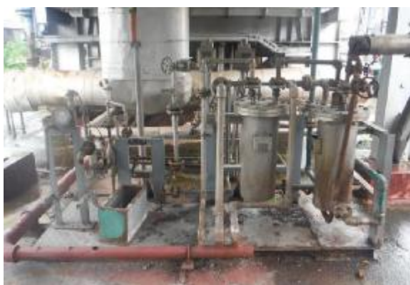
Installed Instrument Failure
