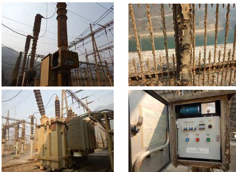
Fig. 3-34 Switchyard Dirt Condition Photos
