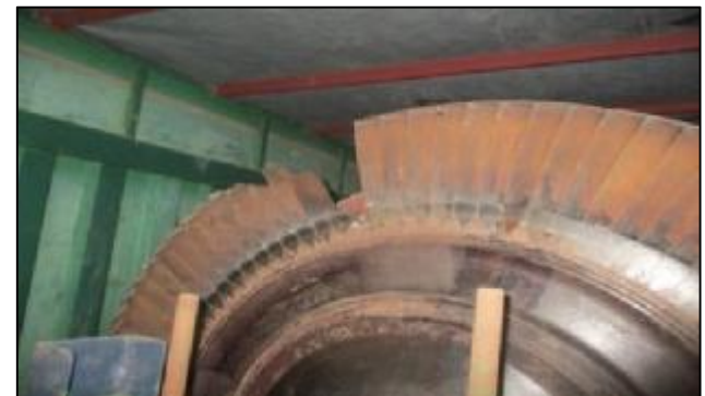
Gas turbine rotor left in damaged condition
