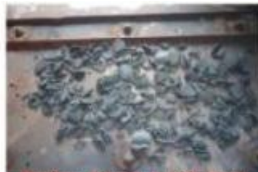
Broken pieces in Exh.Duct
