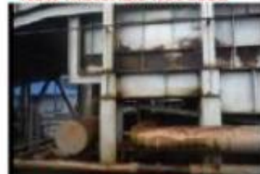
Casing over heated
