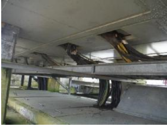
Gas Turbine Common Issue No.3
