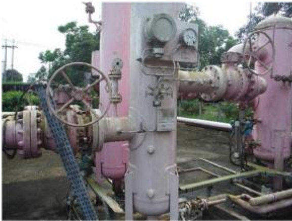
Strainer Inlet/Outlet Flange Gas Leakage
