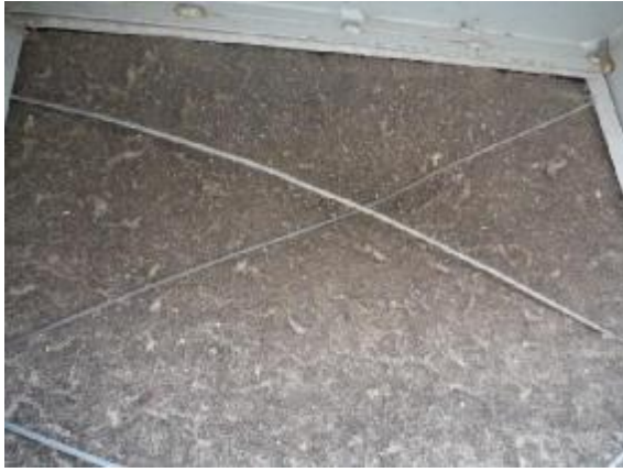
Gas Turbine Common Issue No.1
