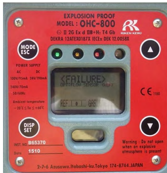
Fig. 4-8 Display of Calorimeter Showing "FAILURE"
