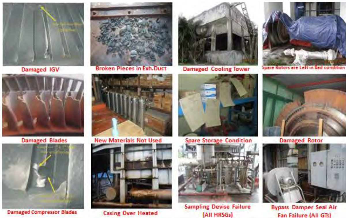
Fig. 3-26 Various Damage (August 2018)
