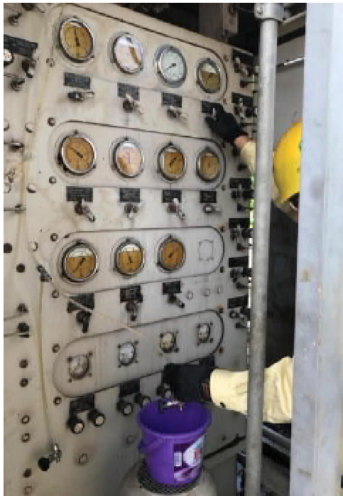
Lube Oil Sampling Sampling Point : #3GT Pressure Gauge Connect point
