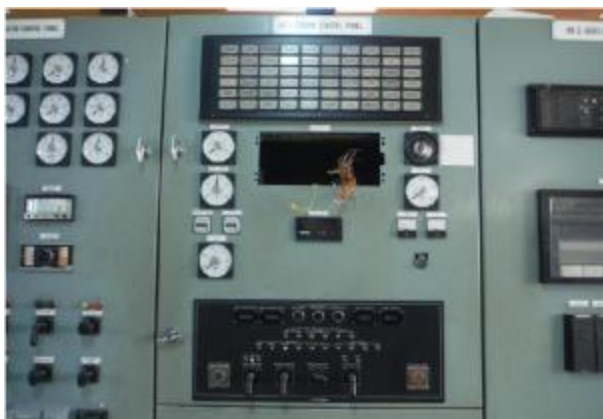
Control and Operation Panel
