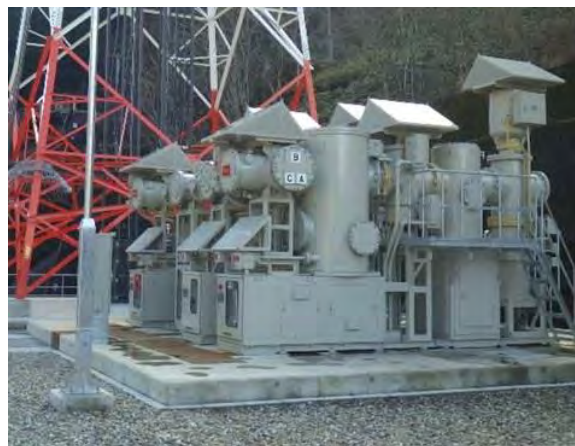
Fig. 5-21 GIS (Gas Insulated Switchgear)
