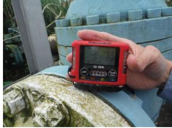
Check Valve Outlet Flange Gas Leakage
