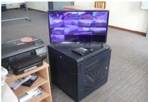
Fig. 3-21 Surveillance Camera Monitoring Screen (Thilawa P/S)
