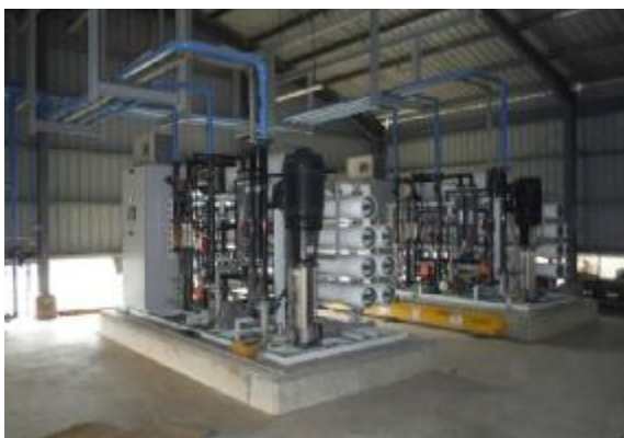
Demineralized Water System
