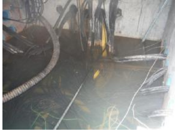
Gas Turbine Common Issue No.4
