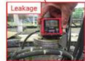
Cyclone separator level gauge lower side flange (32%LEL)
