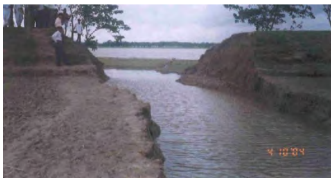
Figure-33 Embankment Breaching
