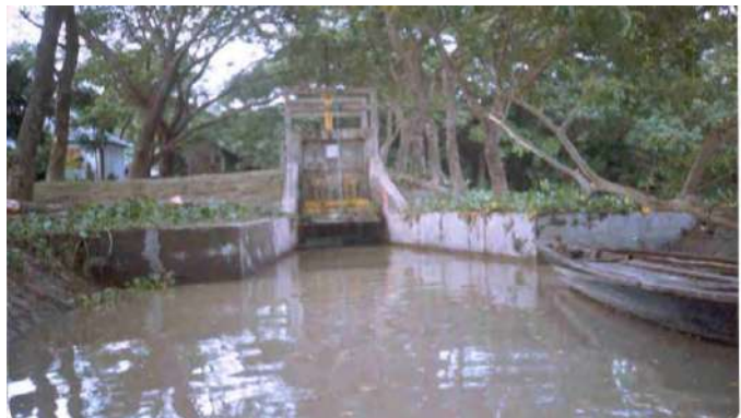
Figure-15 Flap gate lifting system
