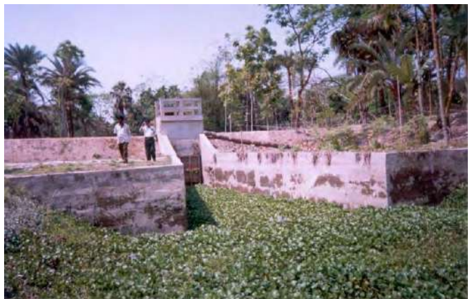
Figure-37 Water Weeds d/S of Structure
