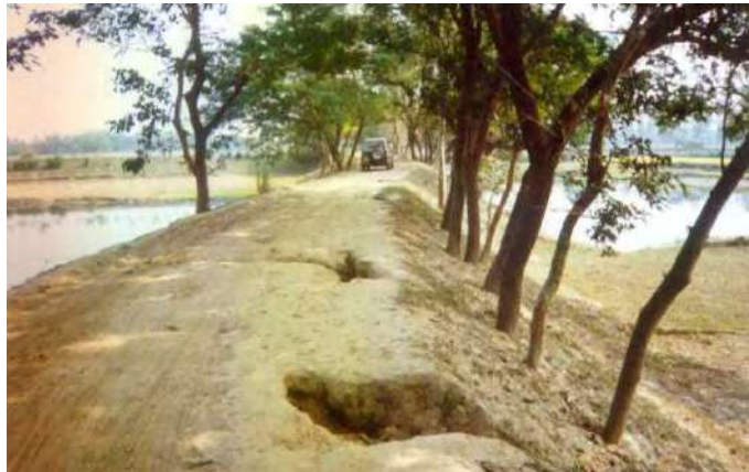
Figure-29 Rut Holes
