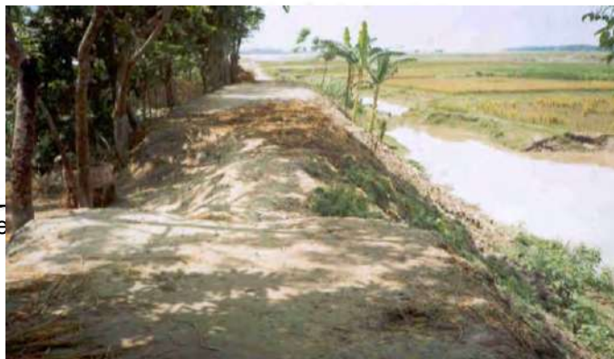
Figure-20 Settlement of Crest and side slope
