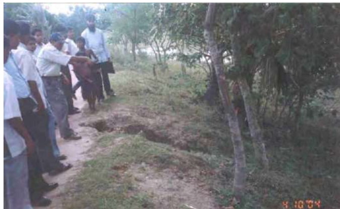
Figure-27 Rain cut
