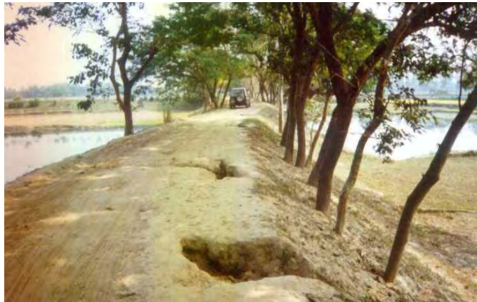
Figure-29 Rut Holes
