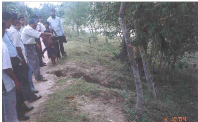
Figure-27 Rain cut
