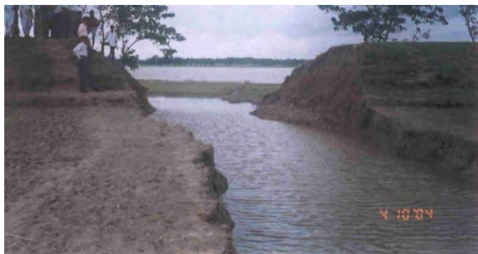
Figure-33 Embankment Breaching
