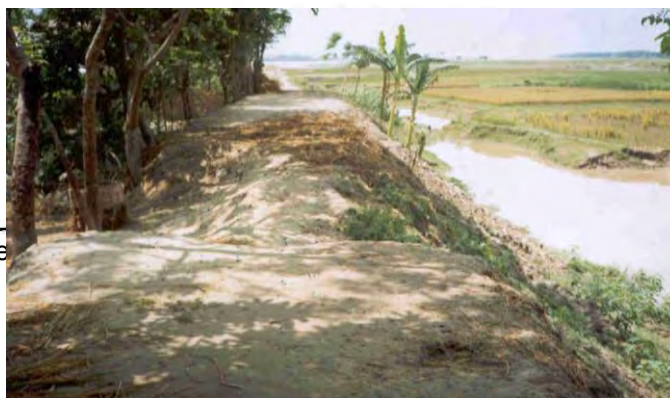
Figure-20 Settlement of Crest and side slope
