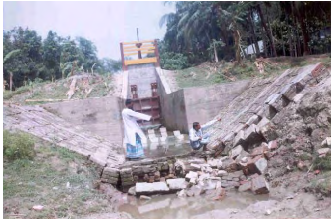
Figure-38 Damage of Protective Works in River Side
