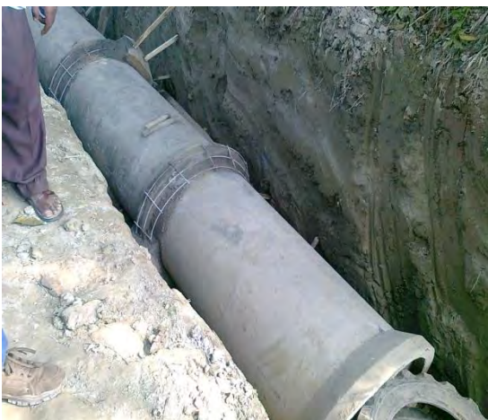
Placement of concrete surround to joints with concrete mortar / bitumen in the joints
