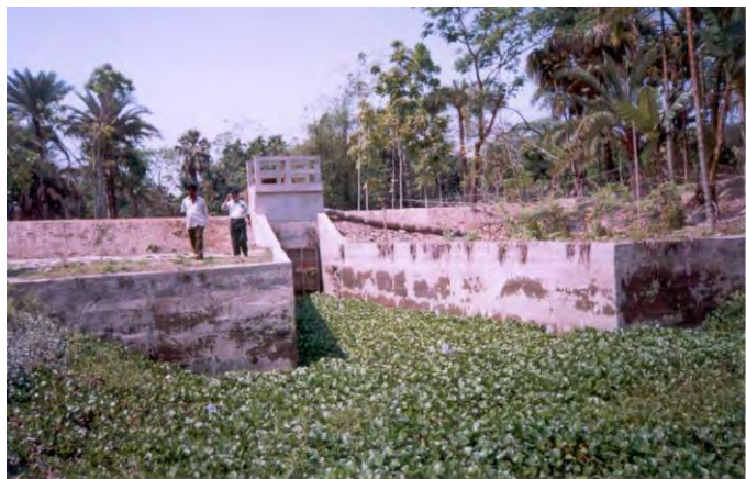
Figure-37 Water Weeds d/S of Structure
