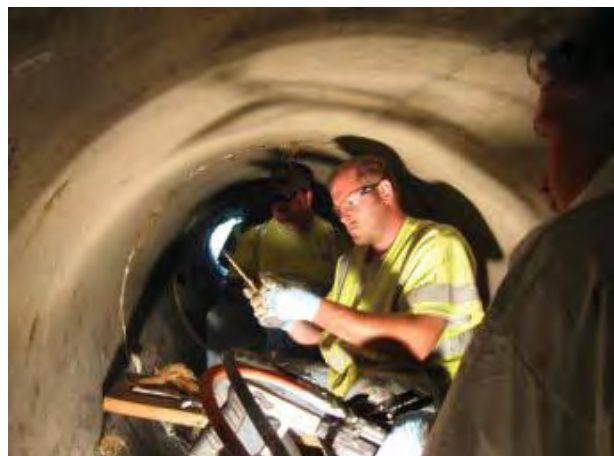
Sealing a pipe joint from the inside with activated oakum (jute fibers soaked with a resin)
