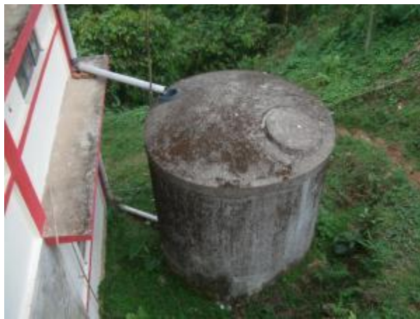
Rain water harvesting tank collecting water from roof top in Bethany Society training center, West Garo Hills District
