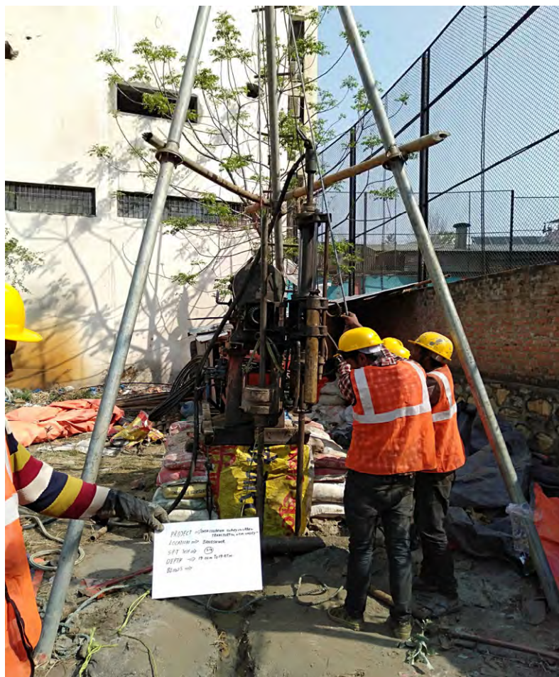
Conducting SPT/DCPT Test for getting (N) Value by Dropping 63.5 kg Hammer from 750mm height
