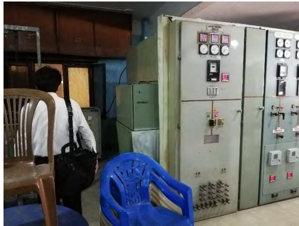
Figure 4.3-11 Space for additional feeder panel
