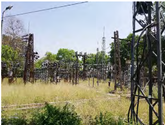
Figure 4.2-36 Old Nepalgunj substation
