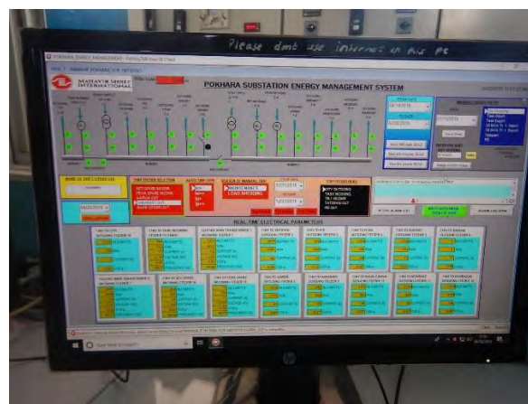
Figure 4.2-3 Monitoring system of 11kV feeders
