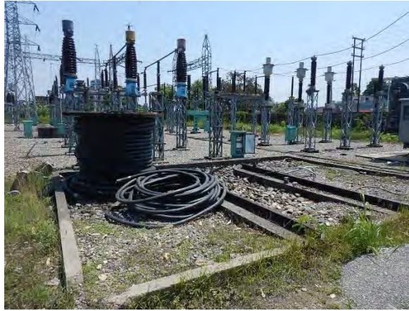
Figure 4.2-4 Future space for additional transformer
