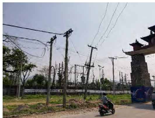
Figure 4.2-12 Outgoing feeders from Pokhara substation
