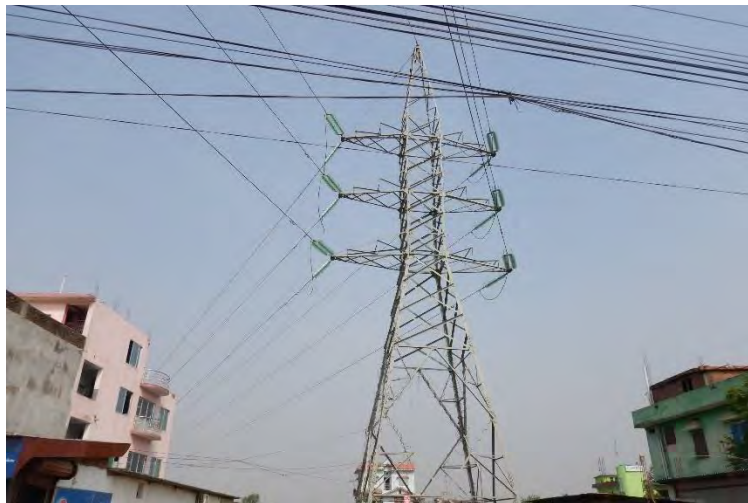
Figure 4.2-24 Tower of the existing transmission line between Kohalpur and Bhurigaon
