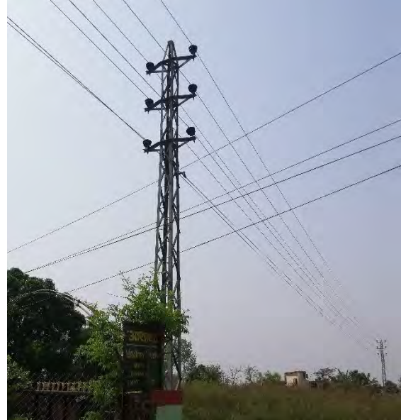
Figure 2.2-8 33kV sub-transmission line
