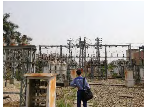
Figure 4.2-37 New Nepalgunj substation
