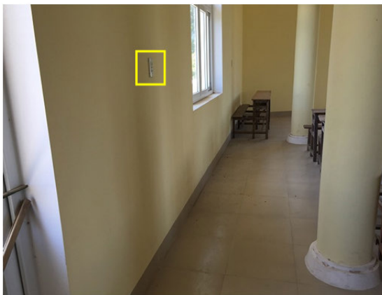
The second floor of the CCCO evacuation center (electric outlet is installed at the upper part of the wall in anticipation for flooding)
