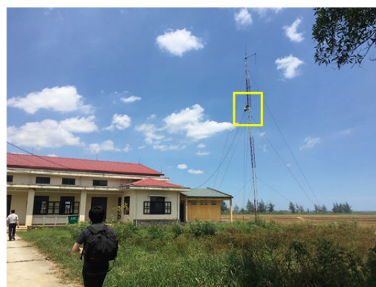
Loudspeaker installed in a commune facility
