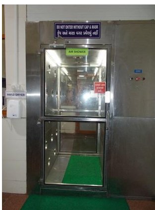
Air shower at cheese production room of Banas dairy
