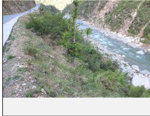
View of slope failure on Valley side:
