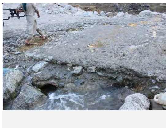
The damage on road has been observed with inlet of pipes for debris flow
