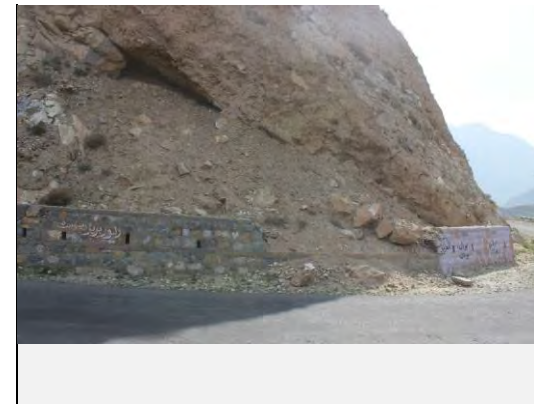
View of unconsolidated material with damaged retaining wall.
