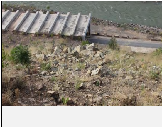
View of landslide on Valley side:
