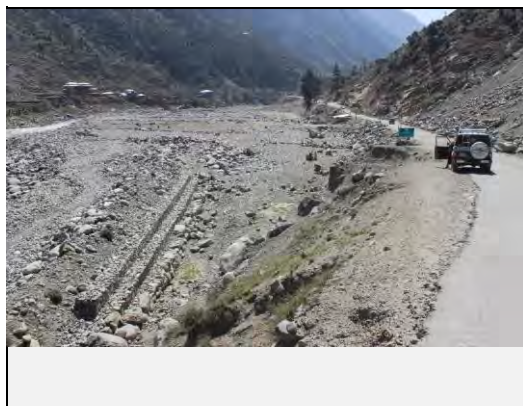
View of slope failure on Valley side and a river diversion structure built at the toe of the slope failure
