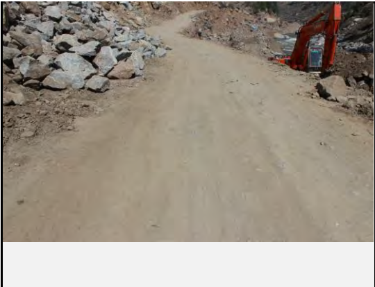
Existing countermeasures / anomalies: Retaining wall is being constructed at the toe of the debris flow
