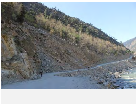
View of the slope failure at the left flank
