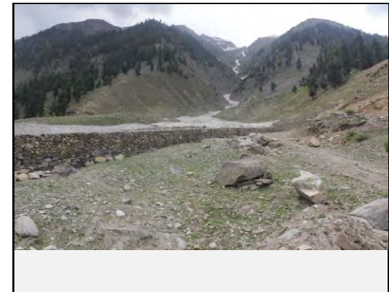
Existing countermeasures / anomalies: Gabion wall has been constructed along the Debris Flow
