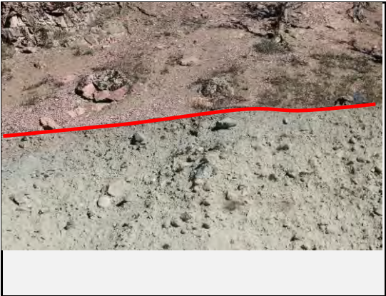
The existing road has been damaged. Red line shows the old road displaced by the debris flow.
