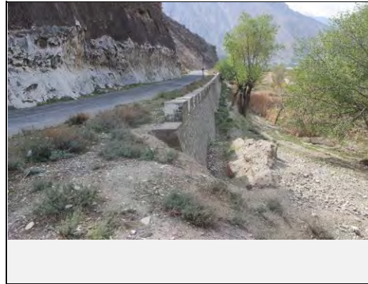
View of Slope Failure on Valley side:
