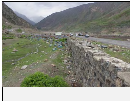
Existing countermeasures / anomalies. Damaged retaining Wall
