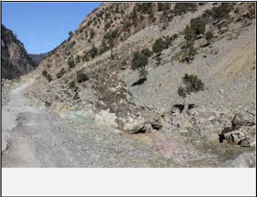
Full view of the slope failure
