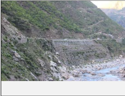
Full view of the slope failure
