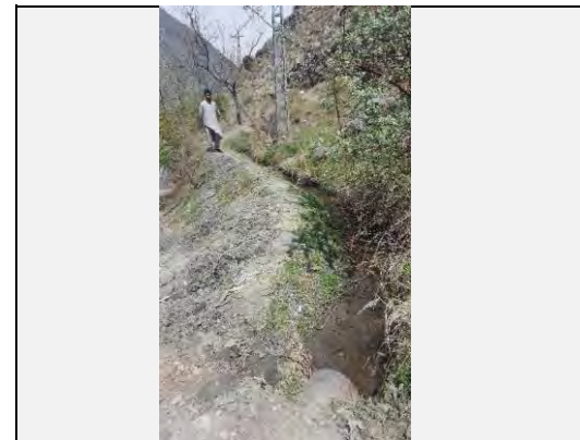
View of water Supply Scheme passing in the middle of the slope failure
