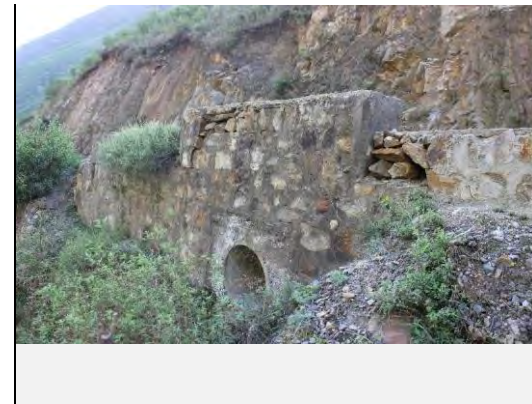
View of Drainage pipe and damaged retaining wall
