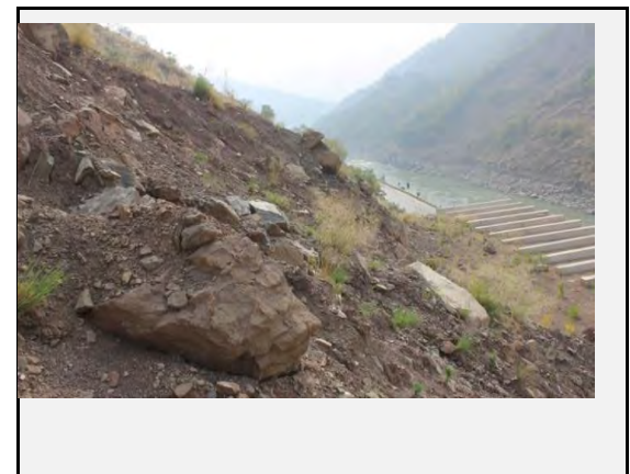
View of fallen blocks on Shed
