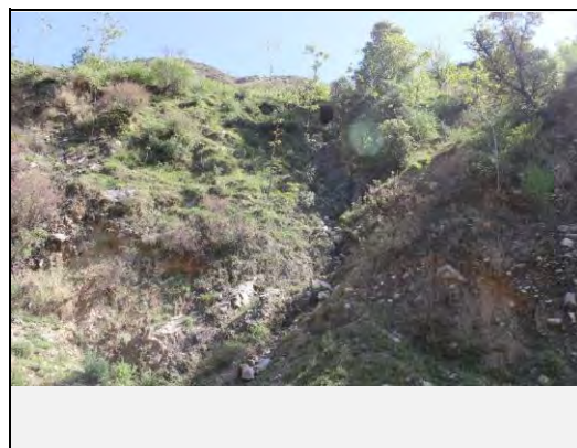
View of Gully erosion along the slope failure
