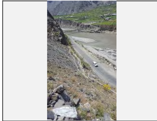
View of slope failure on Valley side:
