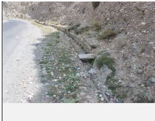
Existing countermeasures / anomalies: View of channel at the toe of Slope Failure
