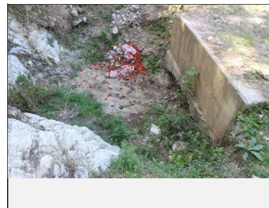
Existing countermeasures / anomalies: View of culvert inlet at the toe of slope failure
