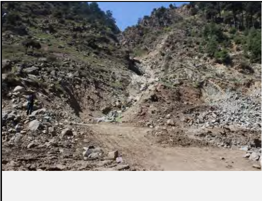
A view of slope failures along the debris flow
