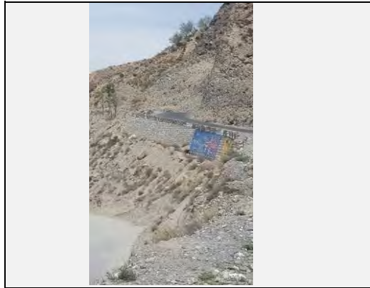
View of Slope Failure on Valley side:
