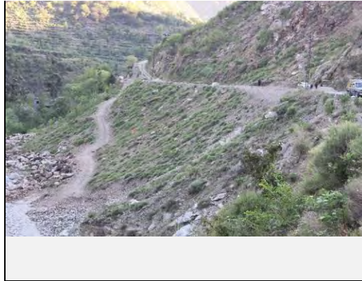
View of slope failure on Valley side:
