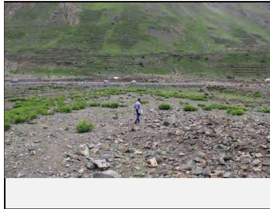
View of Slope Failure on Valley side:
