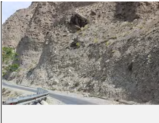
View of the slope failure at the middle point with boulder which threaten the road and traffic.
