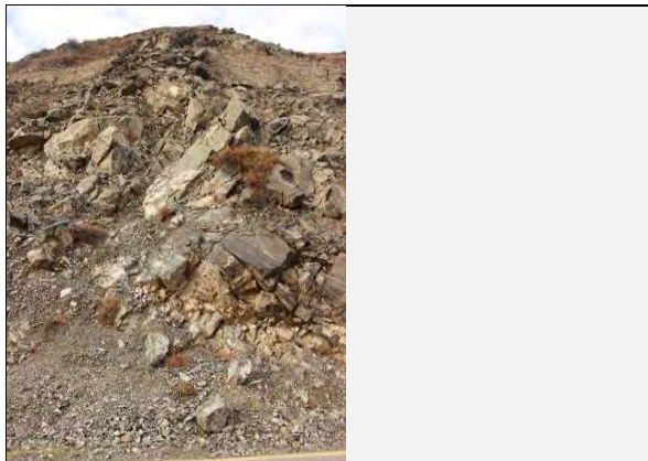
View of the slope failure at the middle point
