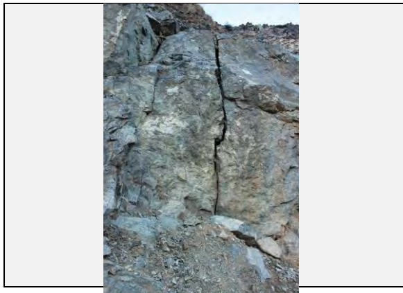
View of the slope failure at the middle point
