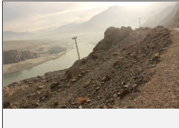
View of landslide on Valley side:
