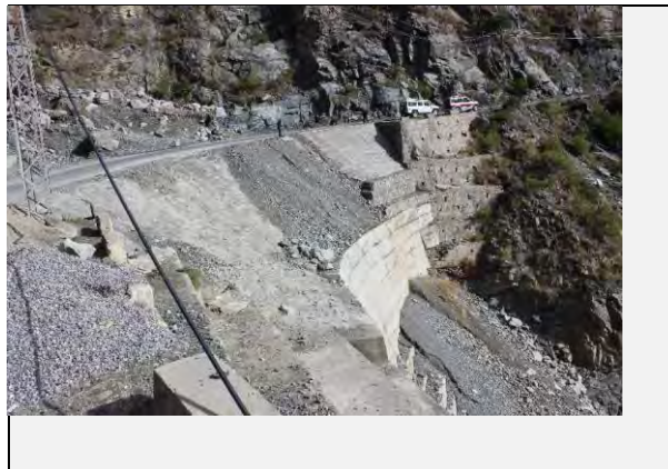
Existing countermeasures / anomalies: Sloped Retaining wall has been constructed for Debris material
