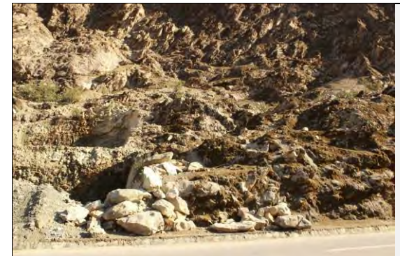
View of fallen blocks
