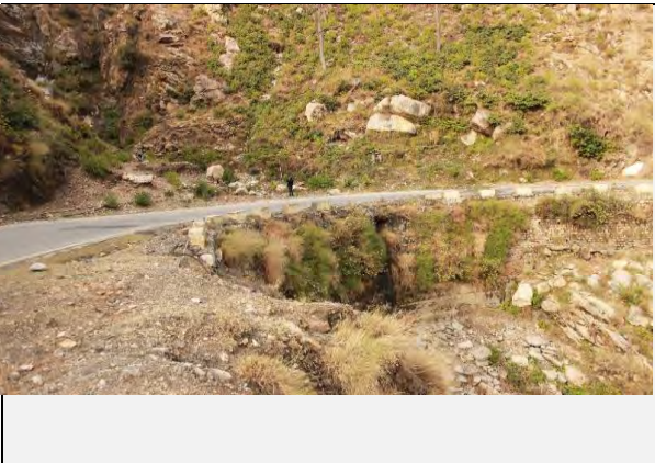
Existing countermeasures / anomalies: Inlet of the culvert is choked by the debris.
