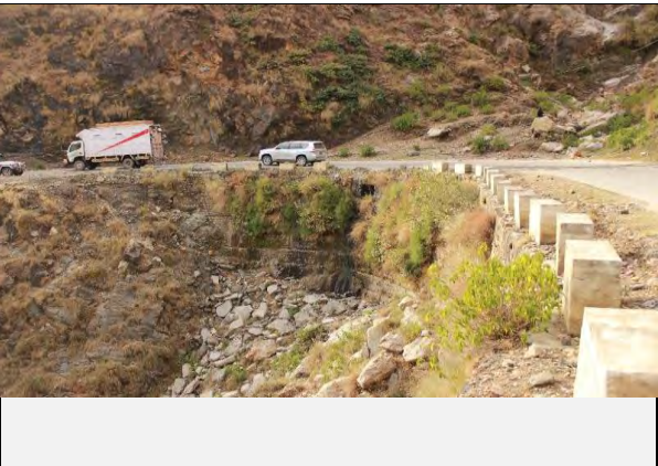
Existing countermeasures / anomalies: Culvert outlet has been constructed at the toe of the debris flow
