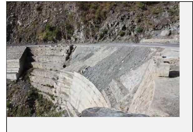
Existing countermeasures / anomalies: Retaining wall has been constructed for N-35
