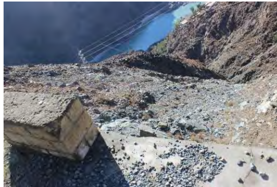
View of landslide on Valley side:
