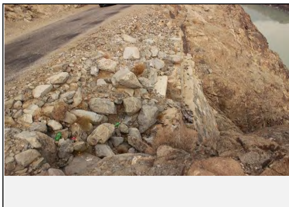
Valley side view of the debris flow
