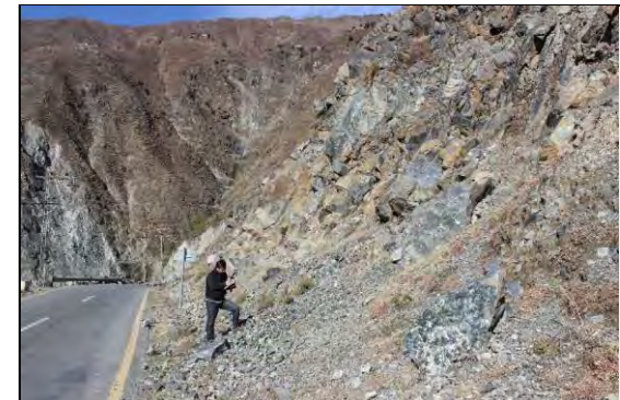
View of Large blocks fallen and talus deposit at the toe of Sloape Failure
