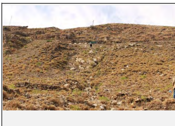
Existing countermeasures / anomalies: View of Culvert outlet as counter measure and retaining wall for N-35
