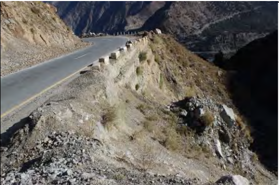
Existing countermeasures / anomalies: View of Retaining wall as counter measure for N-35
