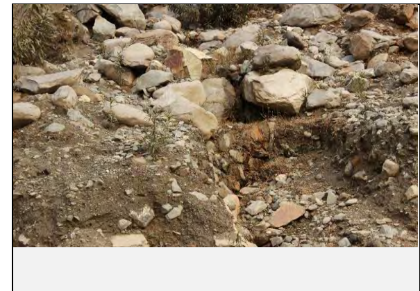
View of fallen blocks along slope failure
