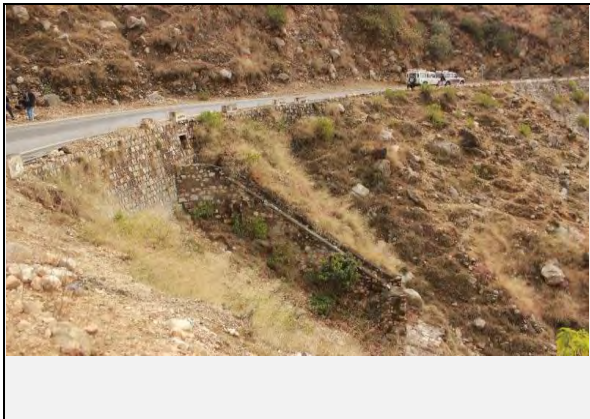
Existing countermeasures / anomalies: View of Culvert as counter measure and retainin wall
