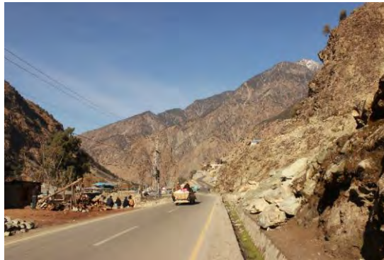
View of landslide on Valley side:
