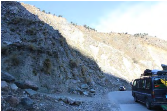
View of the slope failure at the middle point
