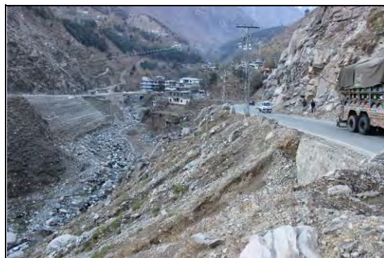
Existing countermeasures / anomalies: View of Retaining wall and benching as counter measure
