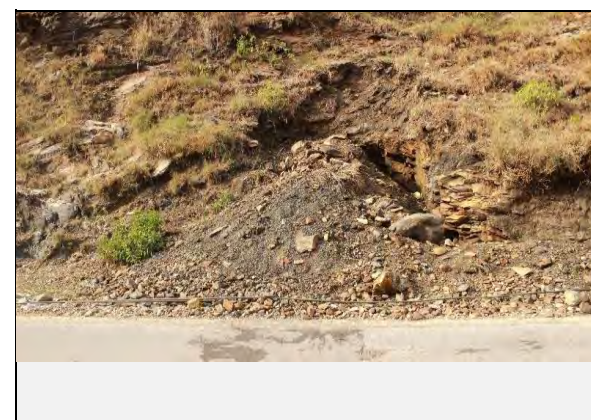
View of new slope failures with the N-35-1
