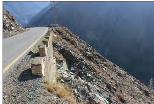
Existing countermeasures / anomalies: View of retaining wall for N-35 as counter measure
