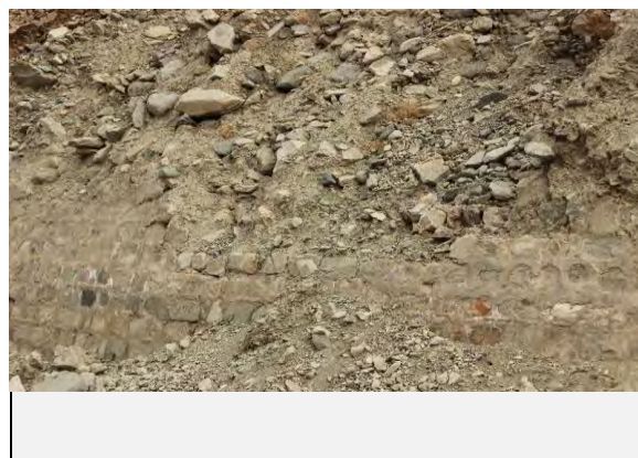
Existing countermeasures / anomalies: View of retaining wall as counter measure for slope failure
