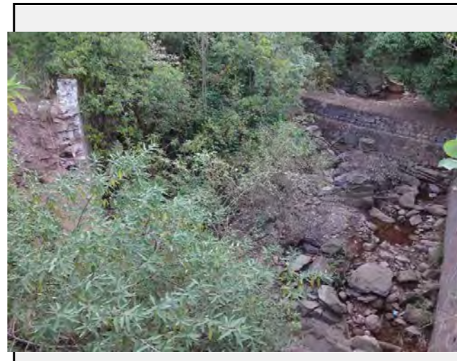
Existing countermeasures / anomalies: Damage on the retaining wall on the north side (undercut slope) on the mountain side.
