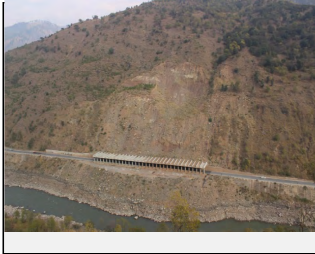
Full view of the landslide
