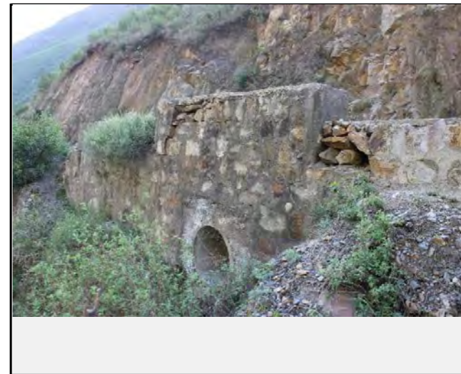
View of Drainage pipe and damaged retaining wall
