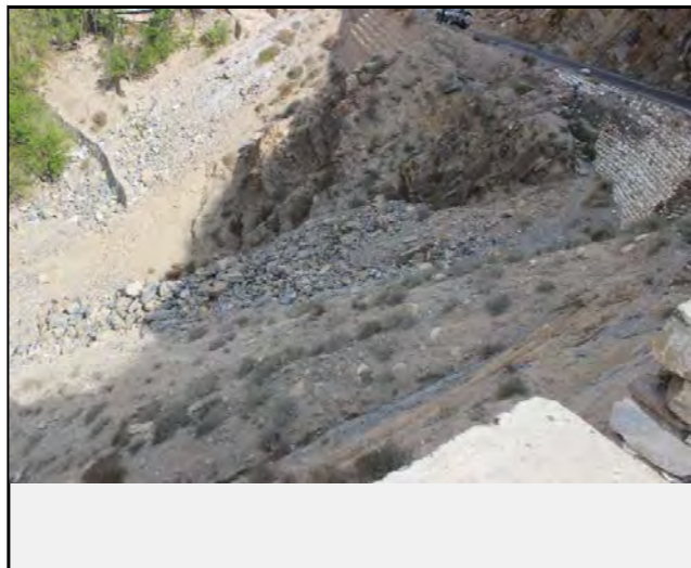
Existing countermeasures / anomalies: View of retaining wall as counter measure for N-45
