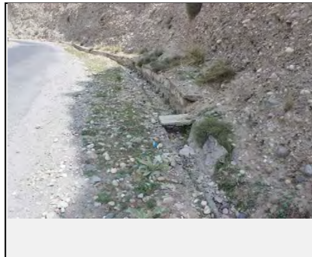
Existing countermeasures / anomalies: View of channel at the toe of Slope Failure
