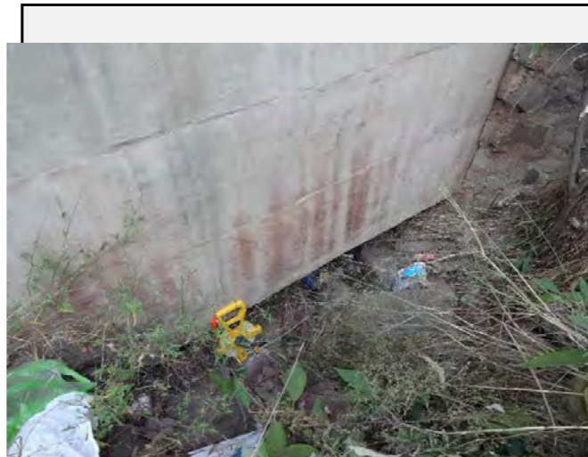
Existing countermeasures: The culvert is filled with debris and rocks which may block the waterway from the mountain area, resulting the flooding of the road.
