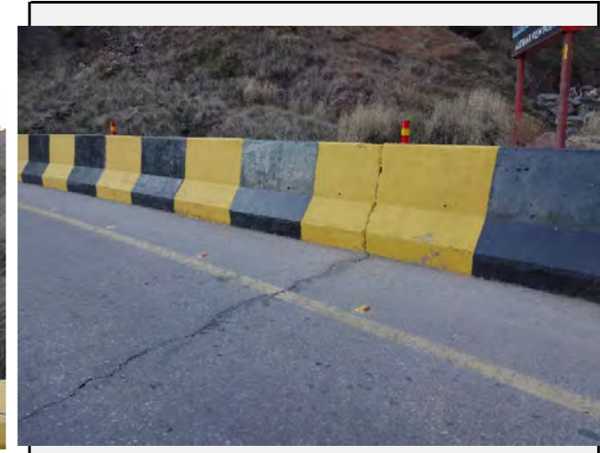
Road condition: Some cracks was observed at the joints of the bridge.
