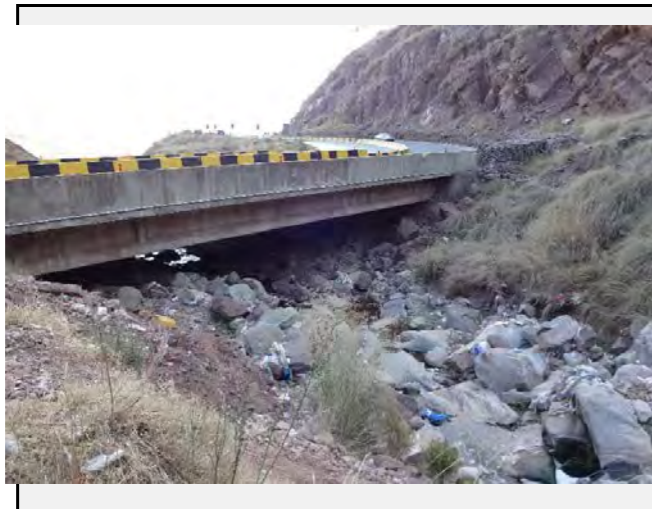
Existing countermeasures / anomalies: Dumping of the garbages around the bridge reduce the capacity to drain the debris to the valley side.
