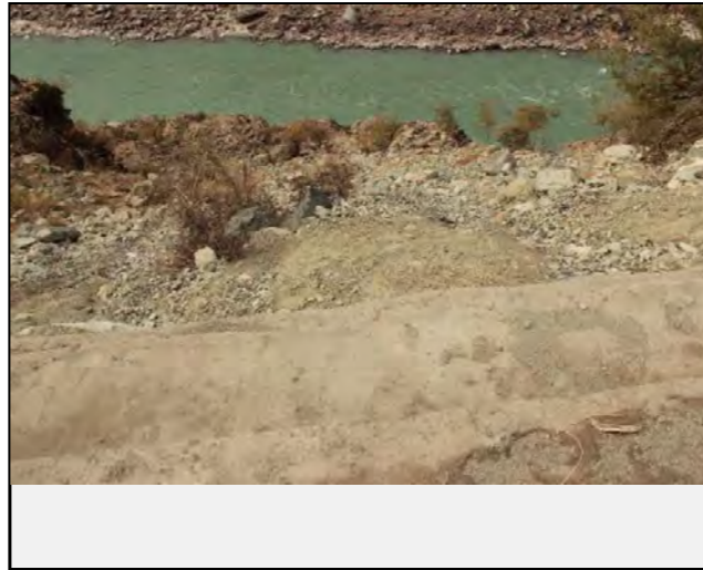
View of slope failure on Valley side:
