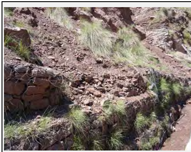
The gabion wall is damaged in many spots due to past rock falls and is thought not to operate properly as a countermeasure
