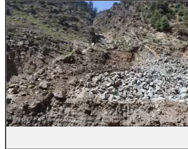
Front view of the debris flow
