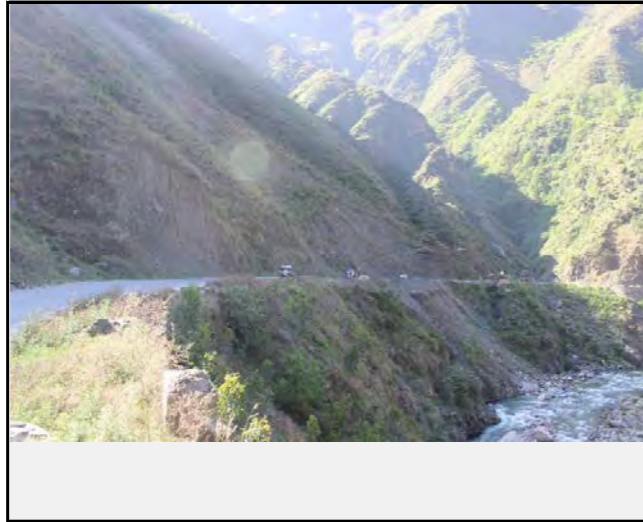
Full view of the landslide
