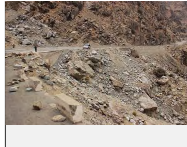
Existing countermeasures / anomalies: Retaining wall has been constructed for N-35
