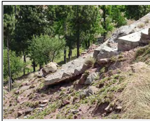
The retaining wall in the valley side is being damaged because the soil on which it is constructed is being washed away.
