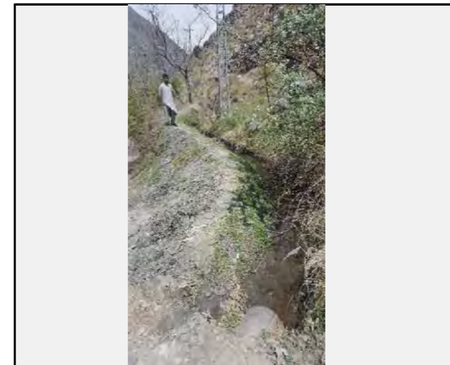
View of water Supply Scheme passing in the middle of the slope failure
