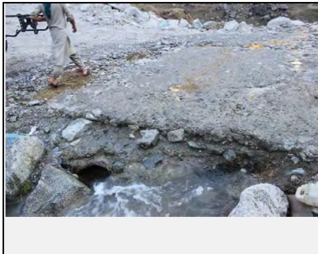
The damage on road has been observed with inlet of pipes for debris flow
