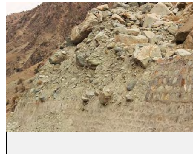
View of fallen blocks
