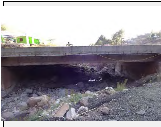
Existing countermeasures : The height underneath the bridge seems enough to clear the debris to the valley side.
