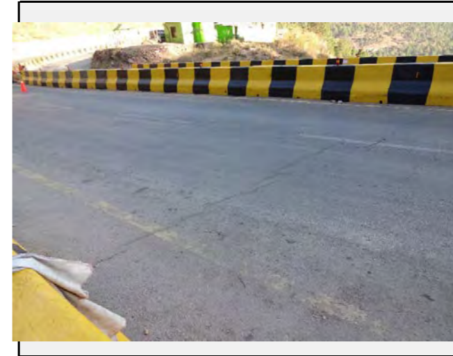
Road condition: Small cracks was confirmed at the joint section of the road and bridge.
