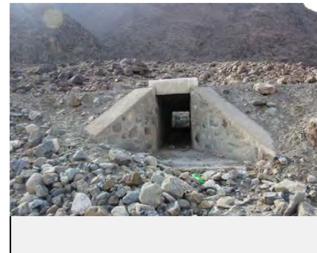
Existing countermeasures / anomalies: Culvert outlet view
