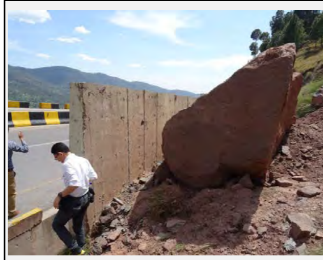
Rock falls of 2m³ have happened in the past reaching the road.
