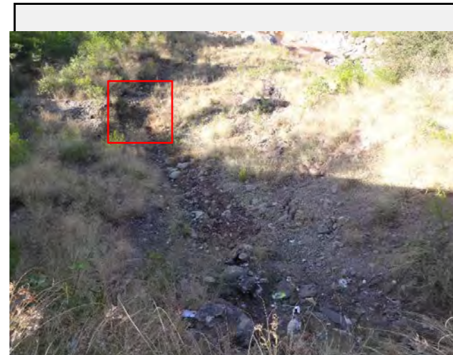
Existing countermeasures: Partial of the gabion works in the valley side was washed away by the debris. Reinforcement of the gabion work will be necessary to stabilize gradient of the river bed.
