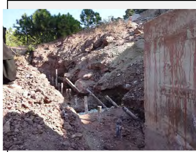
Existing countermeasures / anomalies: Micro piles are installed at the foundation of the lowest retaining wall (ongoing construction).
