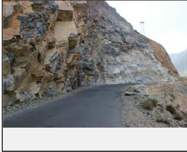
Full view of the landslide
