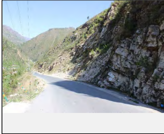
Full view of the landslide
