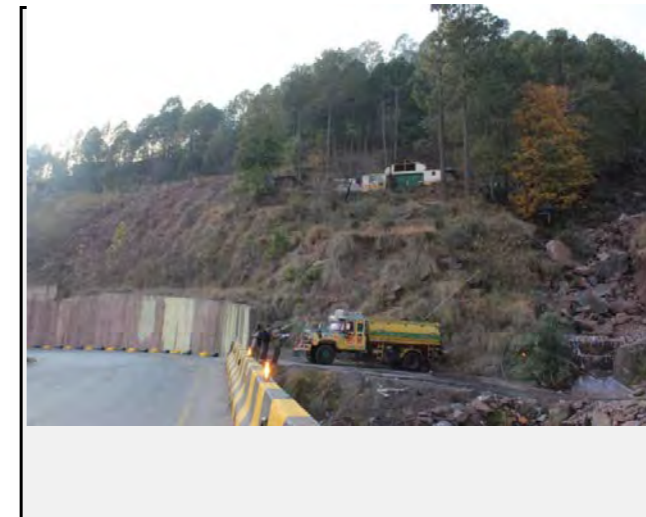
Existing countermeasures / anomalies: Retaining wall has been constructed at the toe of the slope failure
