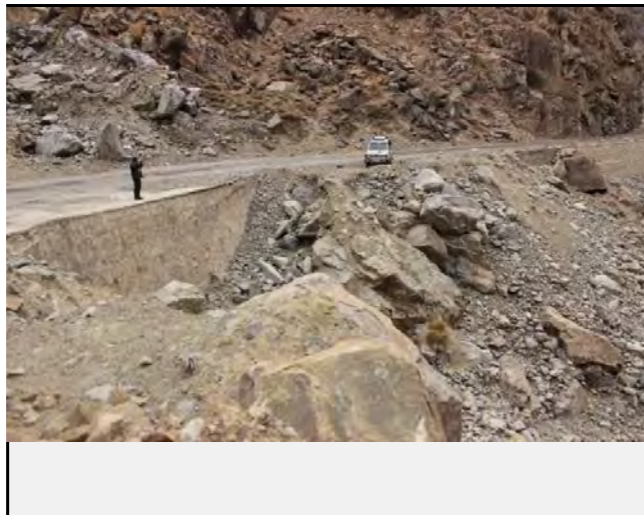
Existing countermeasures / anomalies: Retaining wall has been constructed for N-35 road
