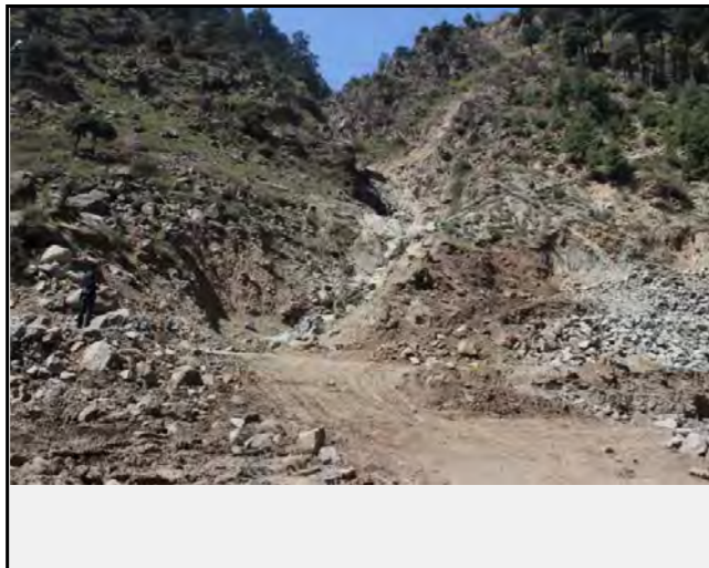
A view of slope failures along the debris flow
