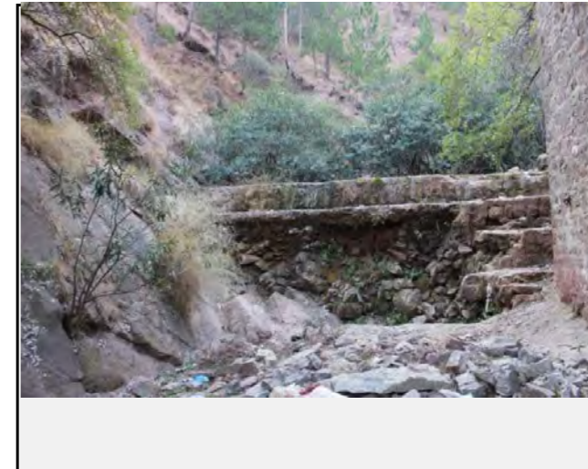
Existing countermeasures / anomalies: Benches has been made on the upstream which are been partially destroyed
