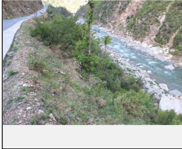
View of landslide on Valley side:
