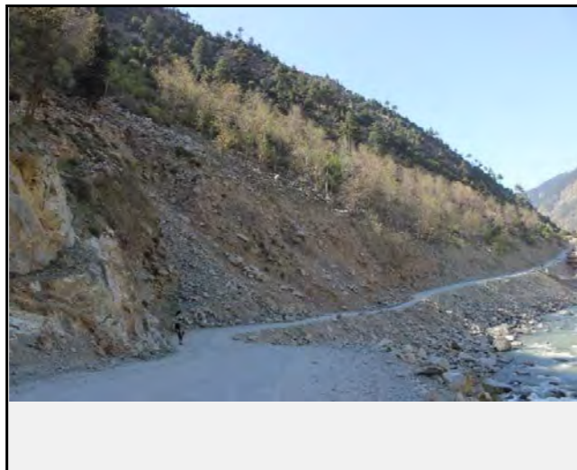
View of the slope failure at the left flank
