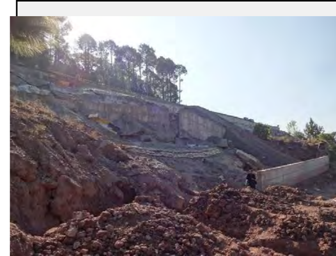
Existing countermeasures / anomalies: Retaining walls are constructed at the valley side of the road (ongoing construction).
