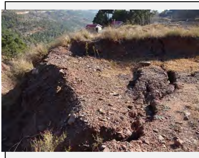
Existing anomalies: Cracks was confirmed on the bank of the valley side. It may collapse in near future due to the erosion.
