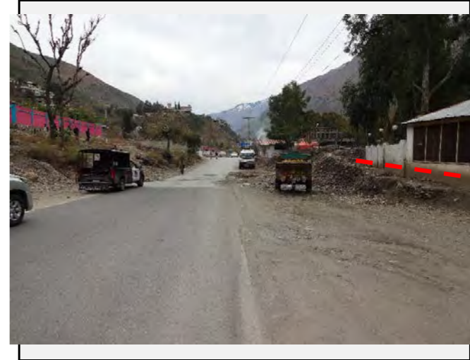
Road condition: Causeway is build on the to allow the stream to flow to the valley side. The red line shows the height of the previous debris flow.
