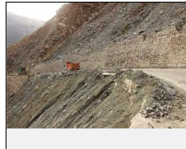
Retaining wall has been constructed to protect the road from the slope failure
