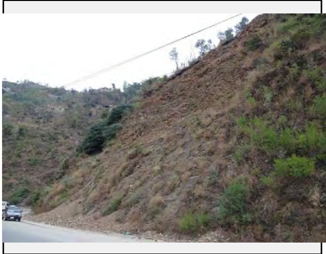
Mountain side: Surface failure was confirmed on the mountain side
