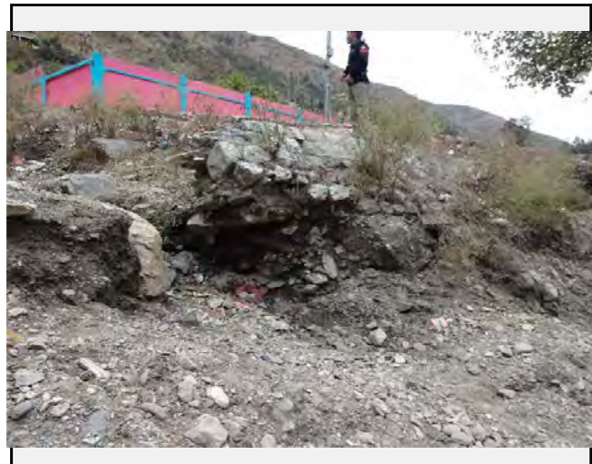
Existing countermeasures / anomalies: Damage of the retaining wall at the exit of the stream
