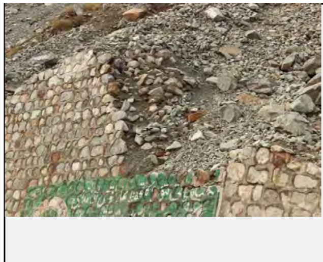
Existing countermeasures / anomalies: Retaining wall has been damaged due to slope failure
