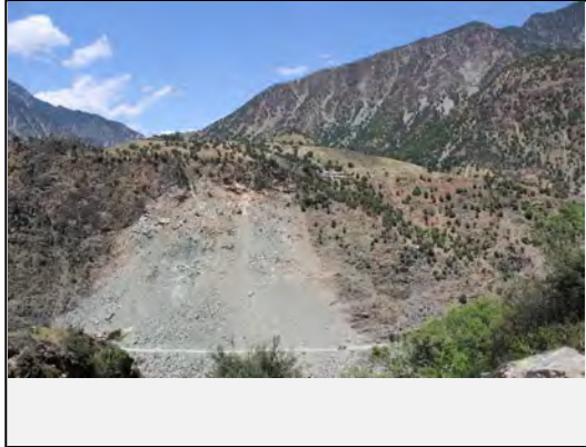
Full view of the Slope Failure
