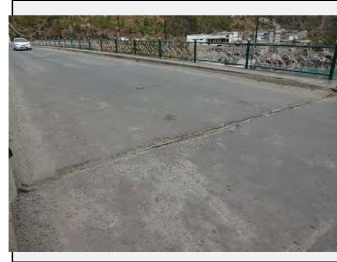
Road condition (old bridge): Some cracks on the boundary of each portion of the suspension bridge.
