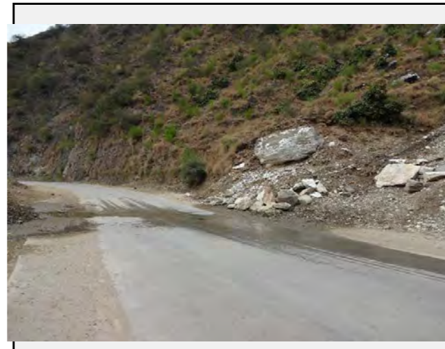
Existing countermeasures / anomalies: Big rock is overhanging just aside of the road. Removal of this rock is recomendable.
