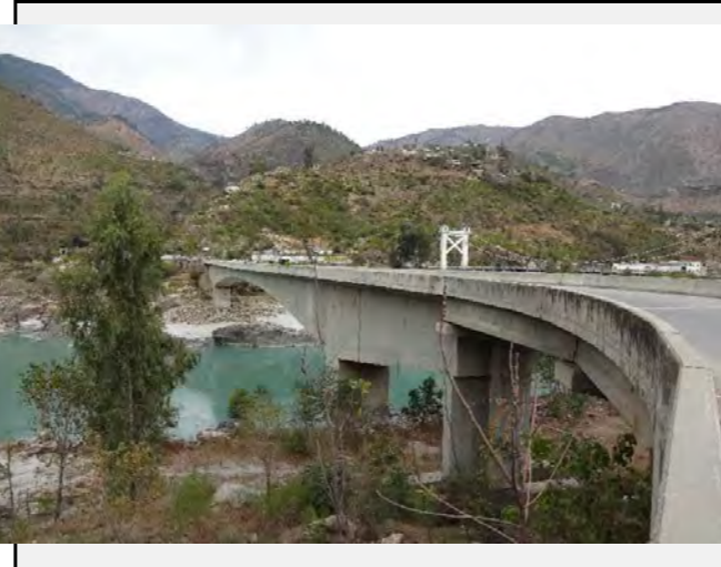
Existing countermeasures: The height of the both bridges is 30m from the water level surface.
