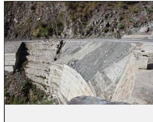
Existing countermeasures / anomalies: Retaining wall has been constructed to protect the road
