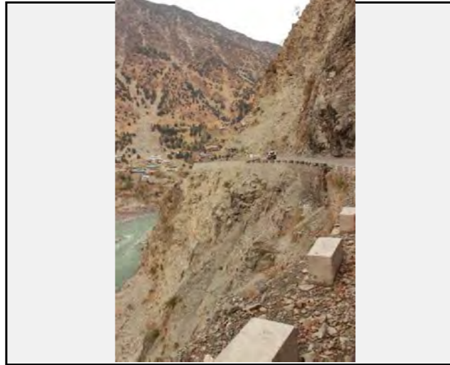
View of the slope failure on Valley side:
