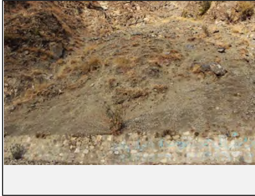
Full view of the Slope Failure
