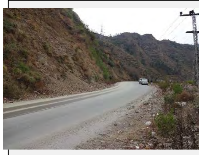
Road condition: No anomalies was confirmed on the road though there are small amount of talus deposited on the shoulder of the road.
