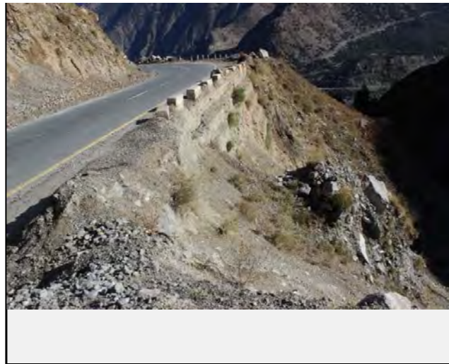
Existing countermeasures / anomalies: View of Retaining wall as counter measure for N-35
