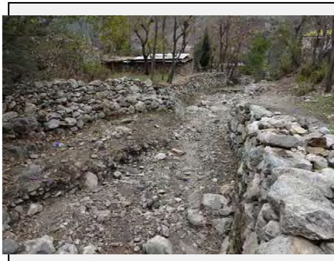
Existing countermeasures / anomalies: The retaining wall by boulders is minimizing the erosion of the bank. However, the stream bed is susceptible to the erosion.
