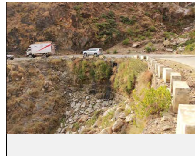
Existing countermeasures / anomalies: Culvert outlet has been constructed at the toe of the debris flow
