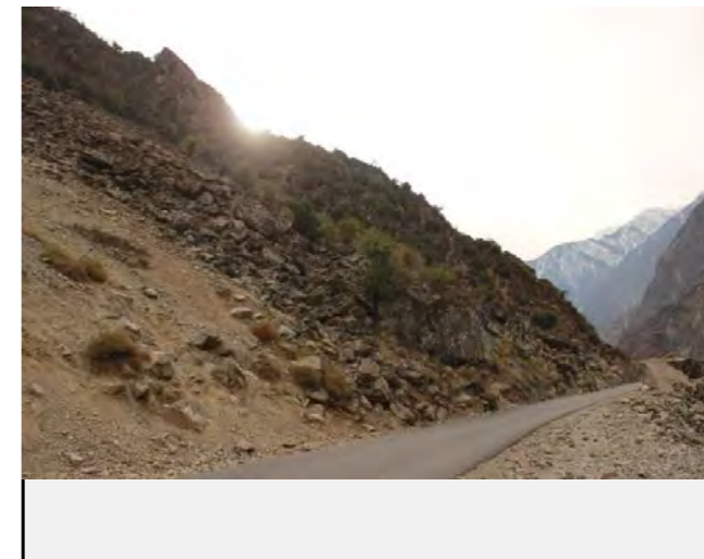
View of fallen blocks
