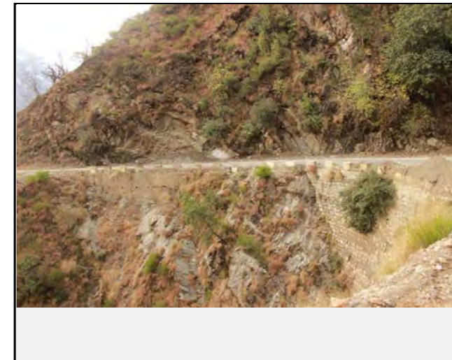
Existing countermeasures / anomalies: Retaining wall has been constructed at the toe of the slope failure
