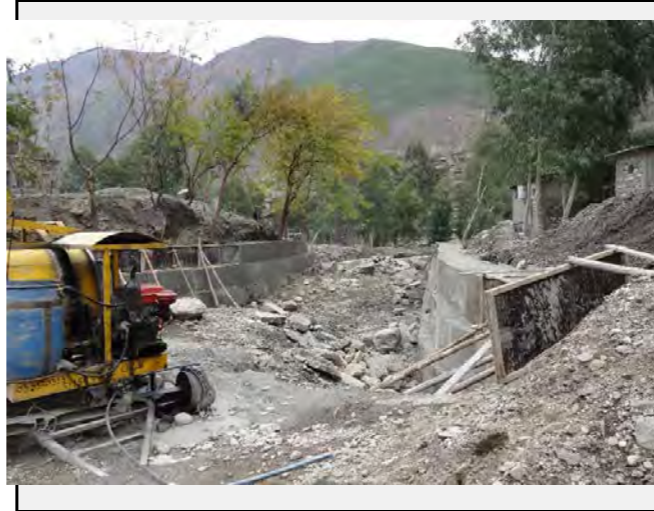
Valley side: Construction of the retaining wall by the inhabitants on the valley side is in progress to protect their houses.
