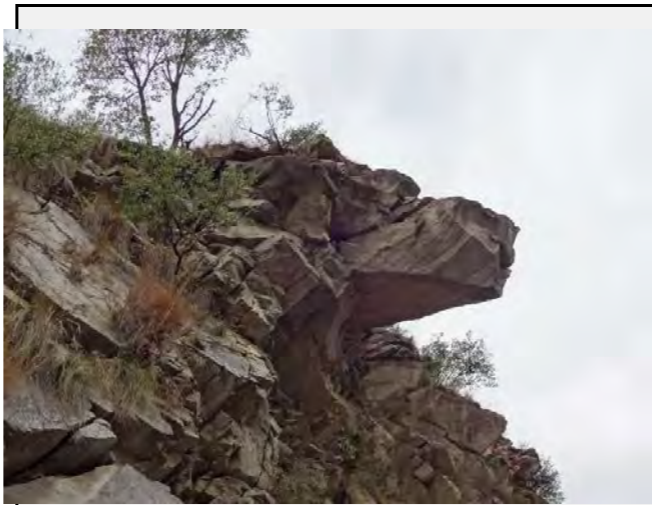
Existing anomalies: Cracks was confirmed on the upper part of the possible falling rock.
