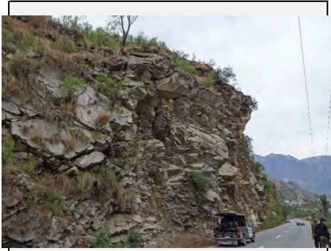
Mountain side: Vertical cut slope along the road is prone to rockfall.
