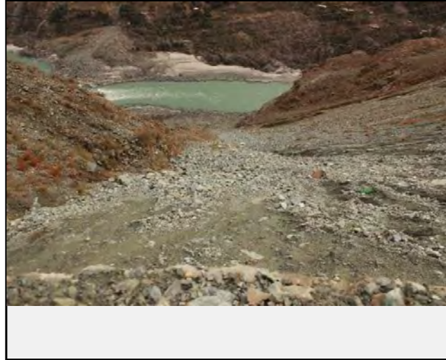
View of slope failure on Valley side:
