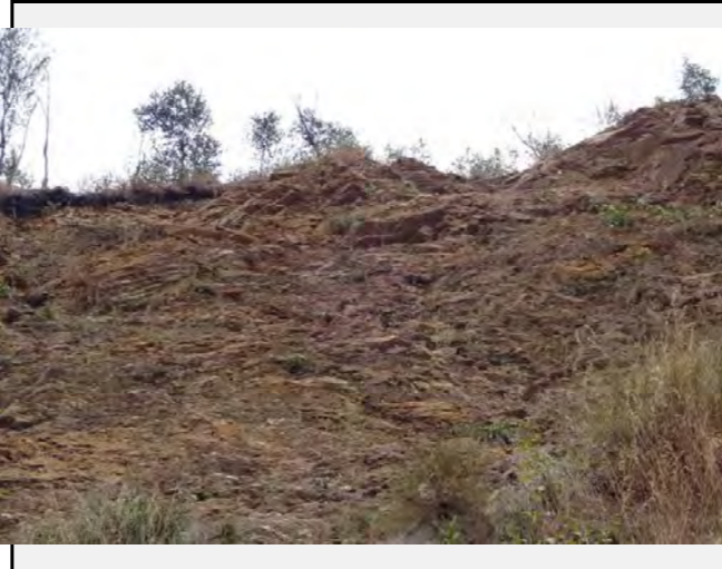
Existing anomalies: Cracks and steep angle accelerate the surface failure.
