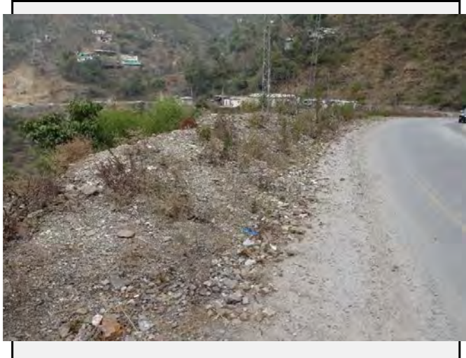
Existing anomalies: The fallen talus deposit is dumped on the valley side of the road.
