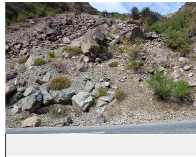
View of fallen blocks along the road
