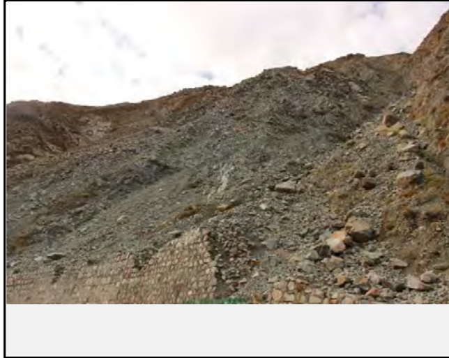
Full view of the slope failure
